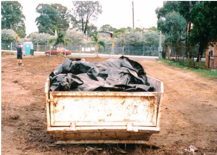
WRAPPED ASBESTOS WASTE
