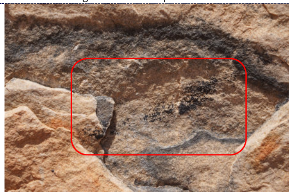
Figure 10: Detail – unknown surface accretion.
