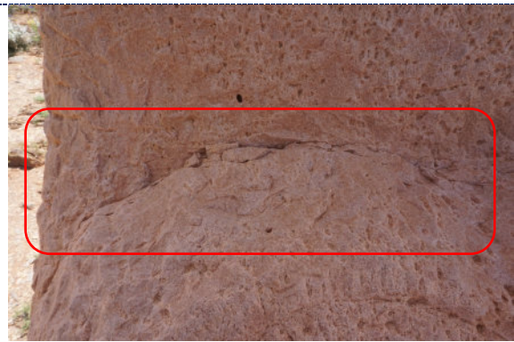
Figure 8: Detail – horizontal crack with minor stone delamination.
