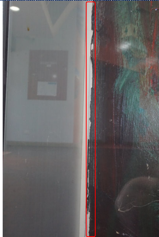
Figure 36: Section 3 – Detail – friable lifting paint layer at edges.
