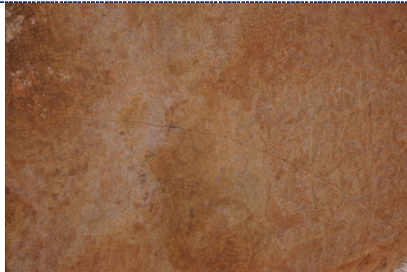
Figure 9: Detail – horizontal crack running through the rear proper right side.
