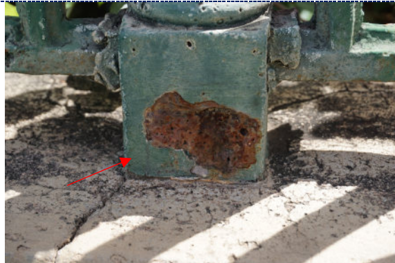
Figure 28: Detail – loss and degradation of green paint on cast iron fencing; iron corrosion product.
