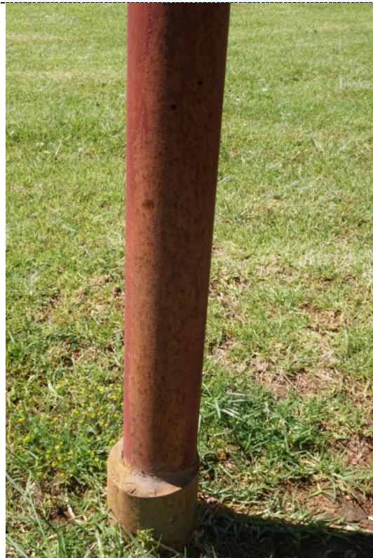
Figure 16: Detail – paint chalking, flaking paint loss with overpaint; corrosion in areas of paint loss; previous repairs (putty/silicone at base).
