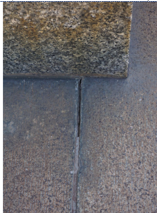
Figure 14: Detail – dirt particulate, red staining (possibly iron corrosion product) and loss to mortar pointing.
