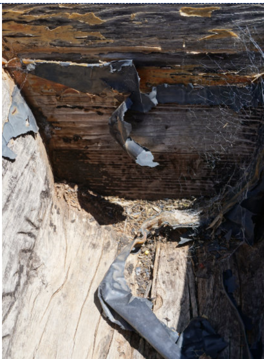
Figure 15: Detail – interior, degraded and peeling varnish, UV degradation (darkening) to wood surface. Interior polypropylene liner, silicon sealant and iron staples heavily degraded. Loose dirt particulate, spider webs and debris.
