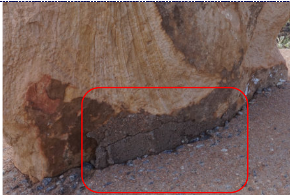
Figure 7: Detail – concrete residue on sandstone.
