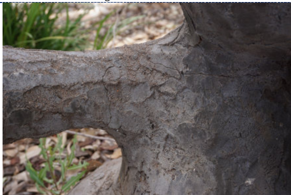
Figure 21: Figure 2 – Detail – dirt particulate, surface cracks.
