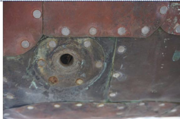
Figure 30: Detail – exterior, dirt particulate, spider webs; corrosion to zinc nail heads; biomatter clogging drains.
