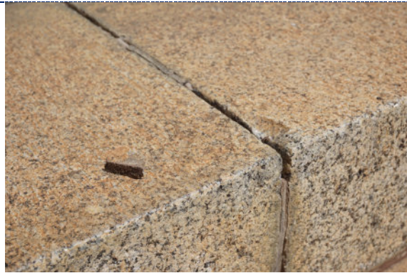
Figure 15: Detail – dirt particulate, red staining (possibly iron corrosion product) and loss to mortar pointing.
