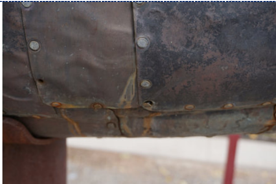
Figure 31: Detail – exterior, missing and loose nail; corroding zinc-iron nails and iron corrosion staining.
