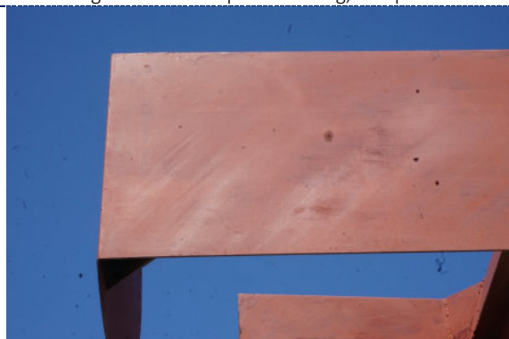
Figure 9: Detail – paint chalking, overpaint.
