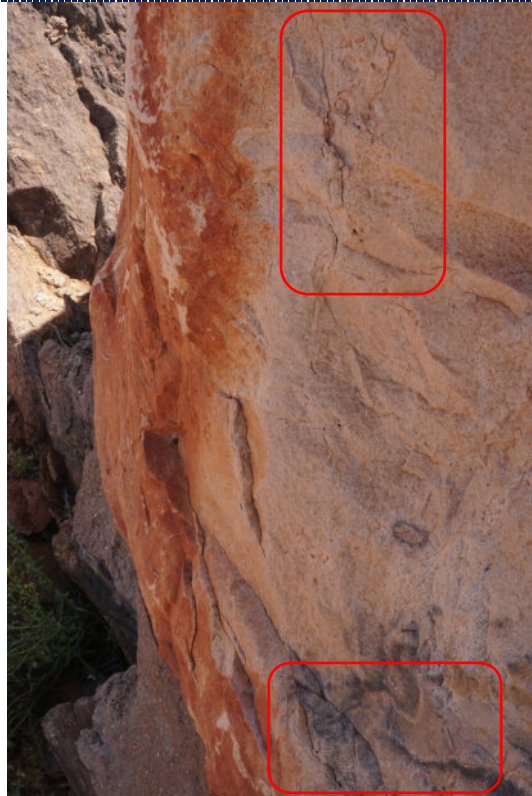
Figure 10: Detail – small cracks, likely occurring naturally in the stone.
