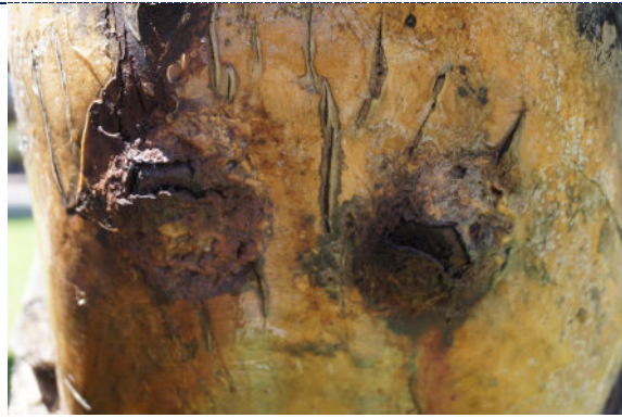
Figure 19: Detail – exterior, corroded iron bolts and peeling varnish.
