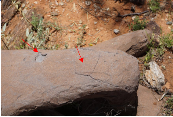
Figure 9: Detail – dirt particulate, large crack and small surface losses.
