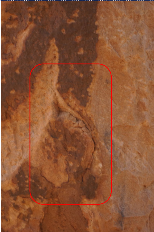
Figure 13: Detail – minor stone delamination.
