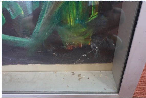
Figure 41: Section 3 – Detail – dirt particulates, surface cracks and spider webs.
