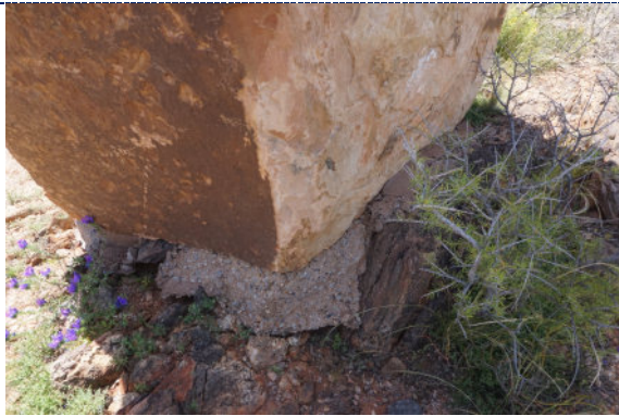
Figure 5: Detail – possible erosion to soil under concrete mortar.
