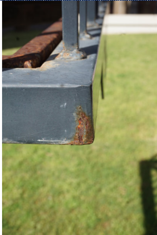
Figure 6: Detail – corrosion occurring at mid-section base piece where paint layer has chipped. Corrosion of the substrate is causing further lifting of the paint in this area.
