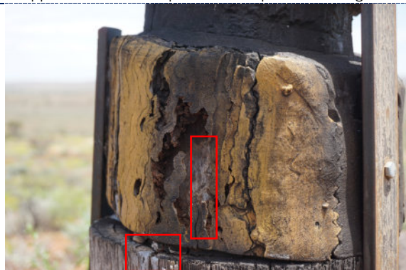
Figure 29: Detail – Pole 4, exterior, UV degradation (darkening) to wood surface, losses to wood likely associated with past insect activity, and presence of bird excrement (highlighted in red).
