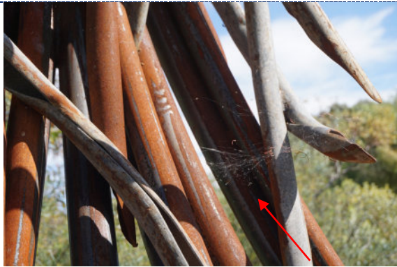
Figure 5: Detail – dirt particulate, spider webs; surface corrosion.
