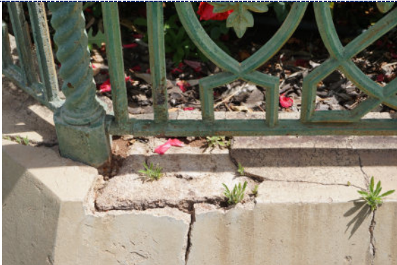
Figure 27: Detail – cracks and loss to plinth render with biogrowth; loss and degradation of green paint on cast iron fencing; iron corrosion product.
