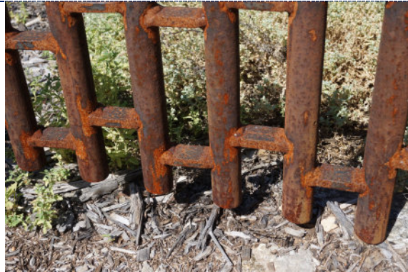
Figure 7: Detail – dirt particulate; surface flash rusting at new welds created during manufacture of artwork.
