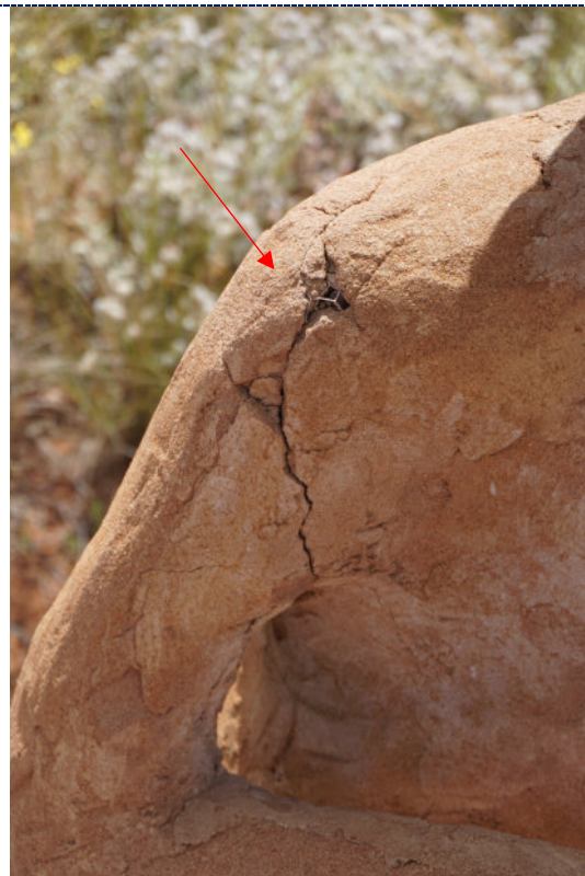
Figure 8: Detail – dirt particulate, large cracks and loss revealing internal iron armature at shoulder.
