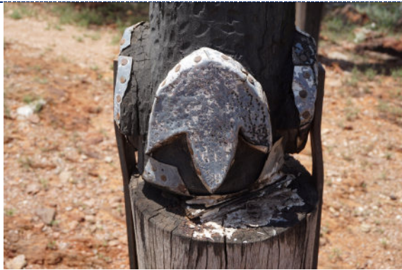
Figure 39: Detail – Pole 6, exterior, UV degradation (darkening) to wood surface, degradation of metal and presence of iron corrosion products. Dirt particulate is present throughout.
