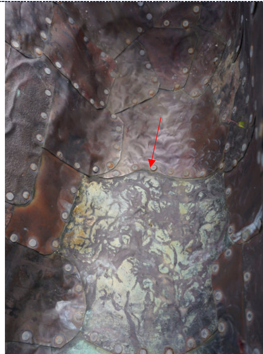
Figure 20: Detail – interior, dirt particulate, green copper corrosion in areas where water pools.
