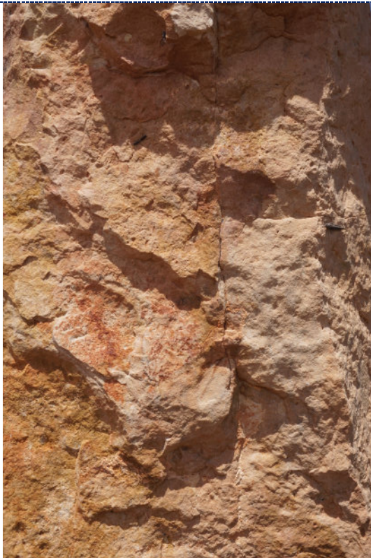
Figure 7: Detail -- vertical crack, likely occurring naturally in the stone.
