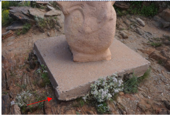
Figure 5: Detail – possible erosion to soil under concrete plinth.
