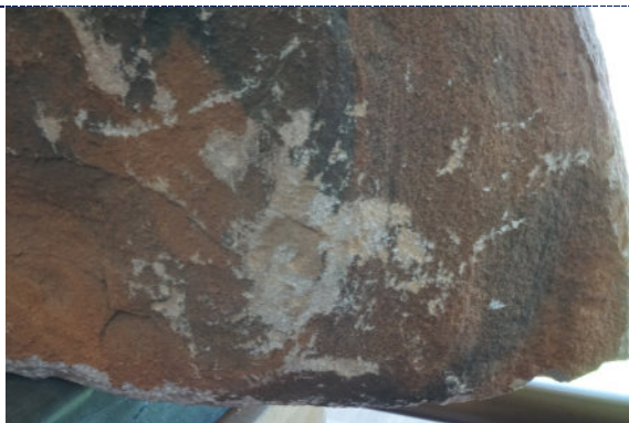
Figure 9: Detail – abrasions with possible stone delamination.
