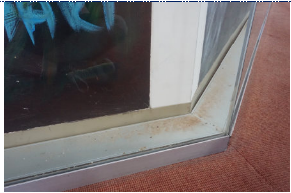
Figure 30: Section 3 – Detail – dirt particulates.
