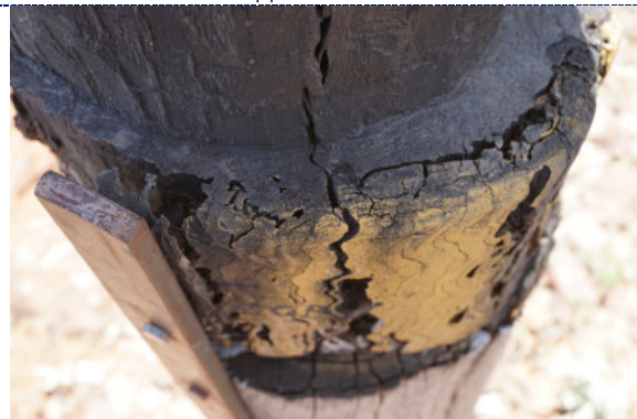
Figure 30: Detail – Pole 4, exterior, UV degradation (darkening) to wood surface, losses to wood likely associated with past insect activity, iron corrosion on metal support brackets.
