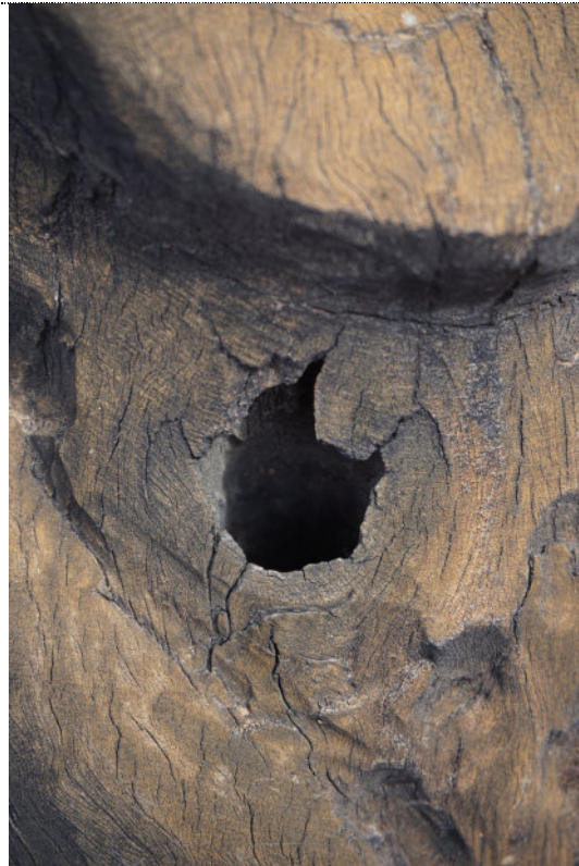
Figure 69: Detail – Pole #2003.0021 Untitled , exterior, UV degradation (darkening) to wood surface throughout. Large loss to the timber pole.
