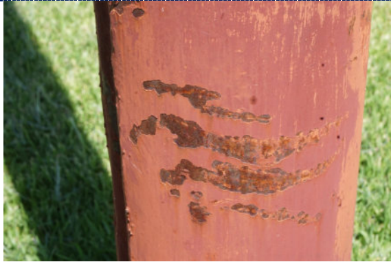
Figure 5: Detail – paint chalking, overpaint; abrasion with loss, likely from contact with foreign object; corrosion in areas of paint loss.
