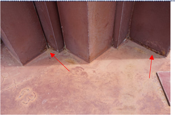
Figure 10: Detail – paint fading and degradation; dirt particulate and surface accretions (white); iron corrosion.
