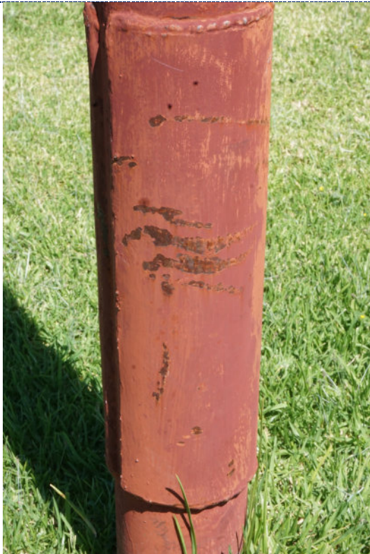
Figure 7: Detail – paint chalking, overpaint; abrasion with loss, likely from contact with foreign object; corrosion in areas of paint loss.
