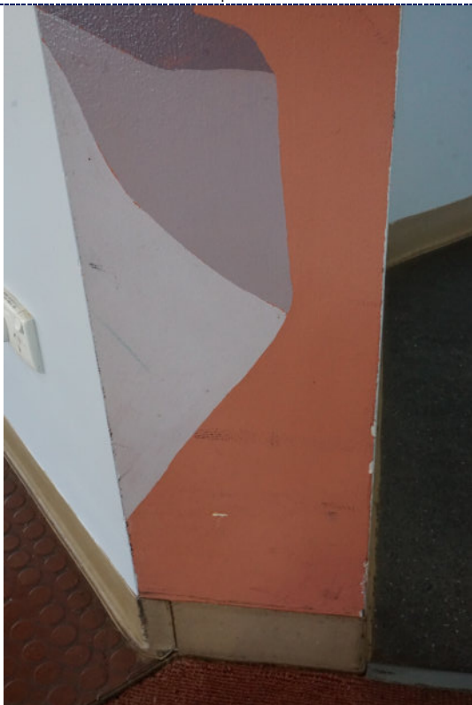
Figure 27: Proper right wall – Detail – surface abrasions with accretions and loss.
