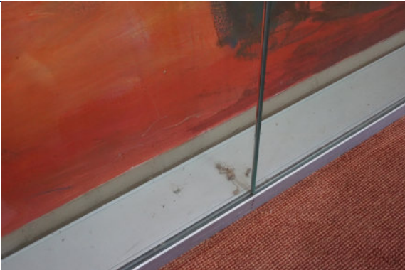
Figure 11: Section 1 – Detail – dirt particulates and spider webs.
