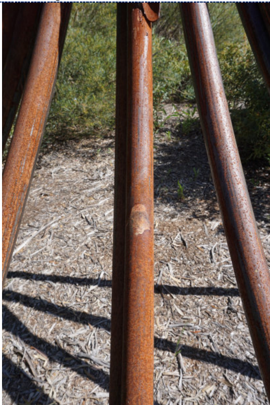
Figure 13: Detail – bird excrement; surface corrosion.
