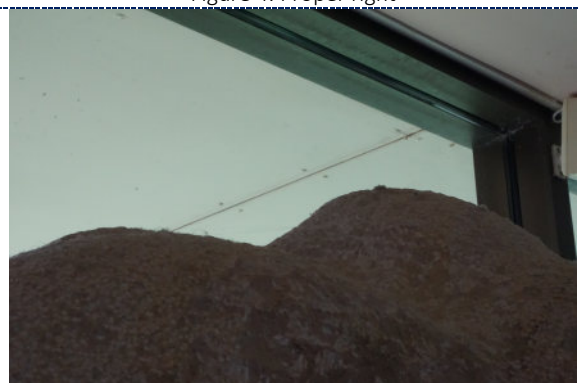
Figure 6: Detail – dirt and dust particulates.
