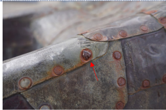
Figure 12: exterior, corroding nail heads and iron staining; one nail head is deformed.
