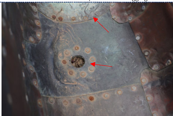
Figure 21: Detail – interior, dirt particulate, green copper corrosion in areas where water pools; biomatter clogging drains.
