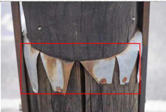
Figure 137: Detail – Pole #2003.0027, Untitled , exterior, iron corrosion and associated staining to the metal body and feathers of the carved bird. The iron staining is highlighted in red.
