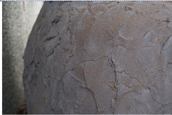
Figure 27: Figure 3 – Detail – dirt particulate, surface cracks.
