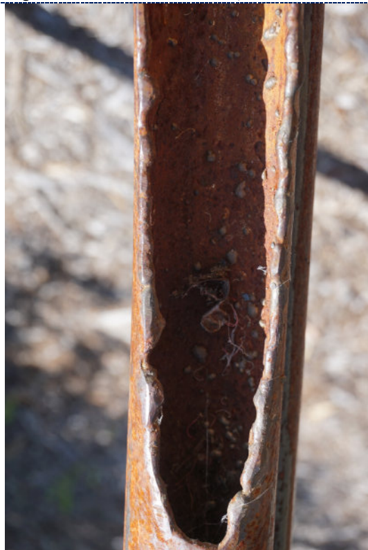
Figure 14: Detail – spider webs; surface corrosion.
