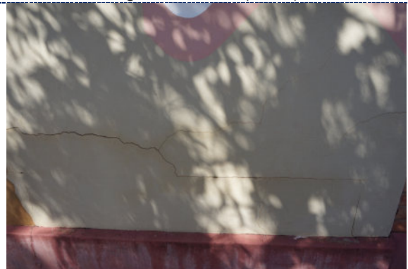
Figure 4: Detail – surface cracks and deformation to the mortar; chalking (UV degradation) and fading of the paint; staining to the exterior of the cracks.
