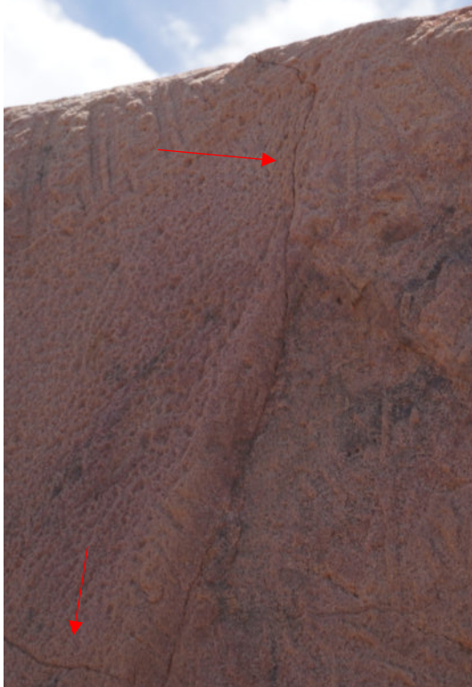
Figure 13: Detail – horizontal and vertical cracks.
