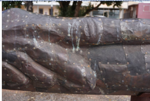
Figure 25: Detail – exterior, dirt particulate; copper corrosion product stemming from bird excrement.
