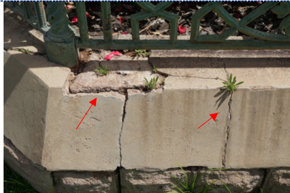
Figure 26: Detail – cracks and loss to plinth render with biogrowth; loss and degradation of green paint on cast iron fencing; iron corrosion product.
