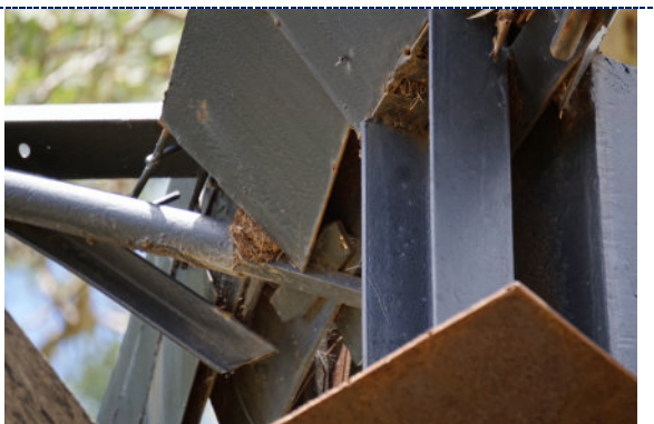
Figure 12: Detail – paint loss and corrosion to iron substrate; accumulated biomatter and spider webs within.
