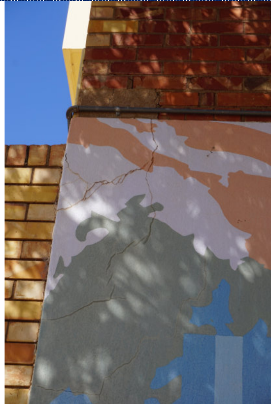
Figure 18: Detail – surface cracks and deformation to the mortar; chalking (UV degradation) and fading of the paint; staining to the exterior of the cracks; small losses.
