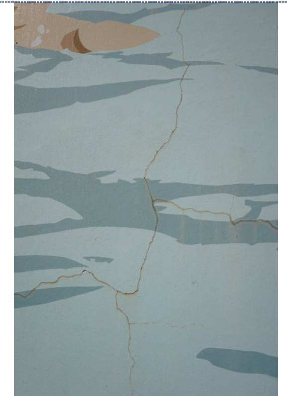
Figure 12: Detail – surface cracks and deformation to the mortar; chalking (UV degradation) and fading of the paint; staining to the exterior of the cracks.
