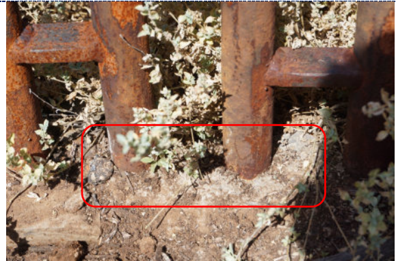
Figure 8: Detail – dirt particulate; surface flash rusting at new welds created during manufacture of artwork; iron inset into concrete.
