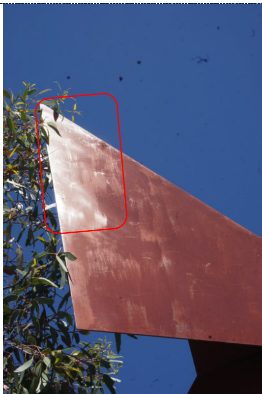
Figure 7: Detail – paint chalking, flaking paint loss with overpaint.
