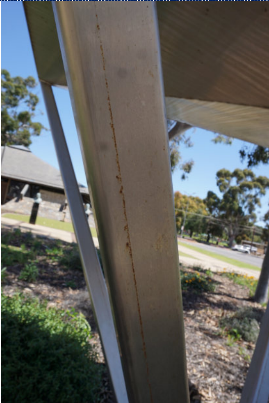
Figure 6: Detail – linear scratch and iron corrosion product.
