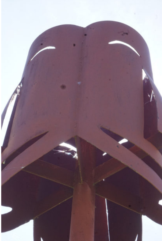
Figure 11: Detail – paint chalking, overpaint; spider webs.
