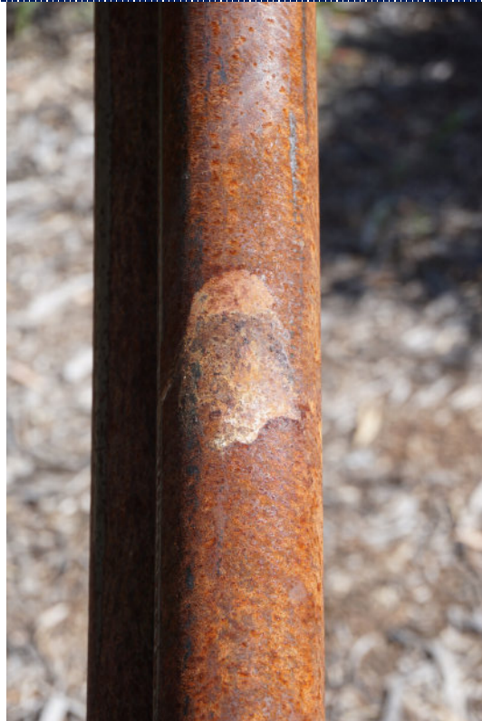
Figure 12: Detail – bird excrement; surface corrosion.
