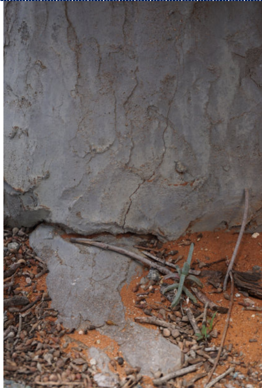
Figure 36: Figure 3 – Detail – dirt particulate, surface cracks.
