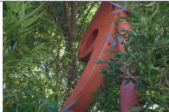
Figure 12: Detail – paint chalking, flaking paint loss with overpaint and corrosion visible.
