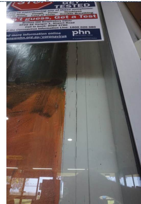
Figure 3: Section 1 – surface cracks.
