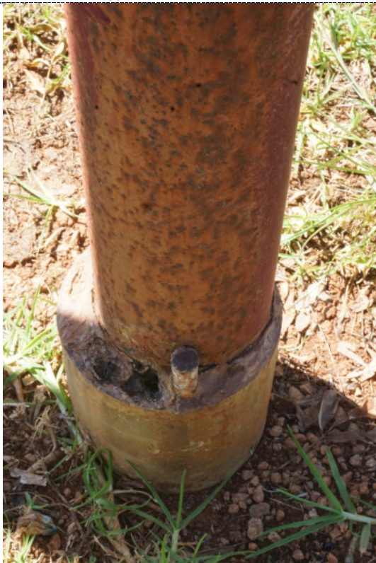
Figure 15: Detail – paint chalking, flaking paint loss with overpaint; corrosion in areas of paint loss; previous repairs (putty/silicone at base).
