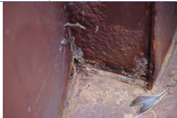
Figure 14: Detail – paint fading and degradation; dirt particulate and surface accretions (white); iron corrosion; dirt particulate, accumulated biomatter and spider webs.
