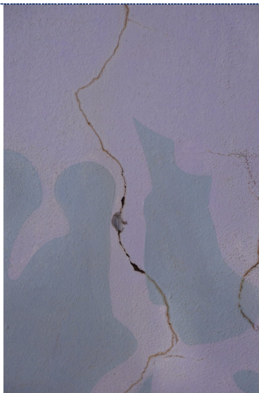
Figure 16: Detail – surface cracks and deformation to the mortar; chalking (UV degradation) and fading of the paint; staining to the exterior of the cracks; small losses.
