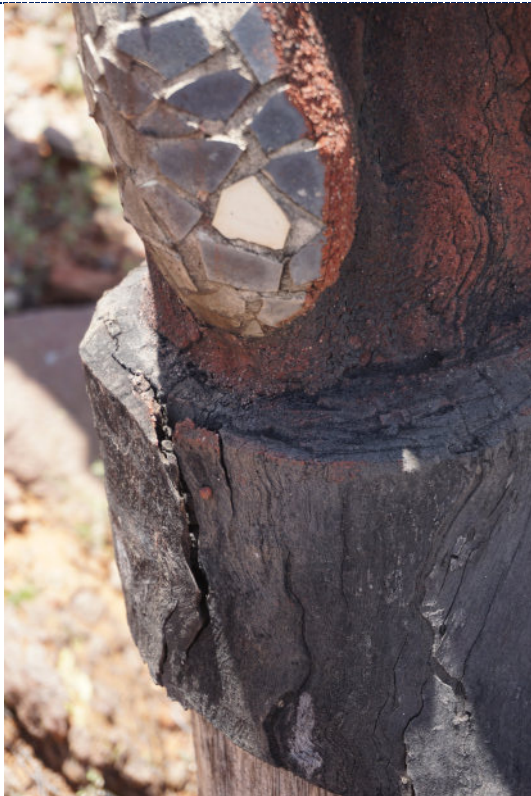
Figure 73: Detail – Pole 10, exterior, UV degradation (darkening) to wood surface, extensive losses to wood and painted surfaces and degradation to the binder securing the mosaic tiles in place.
