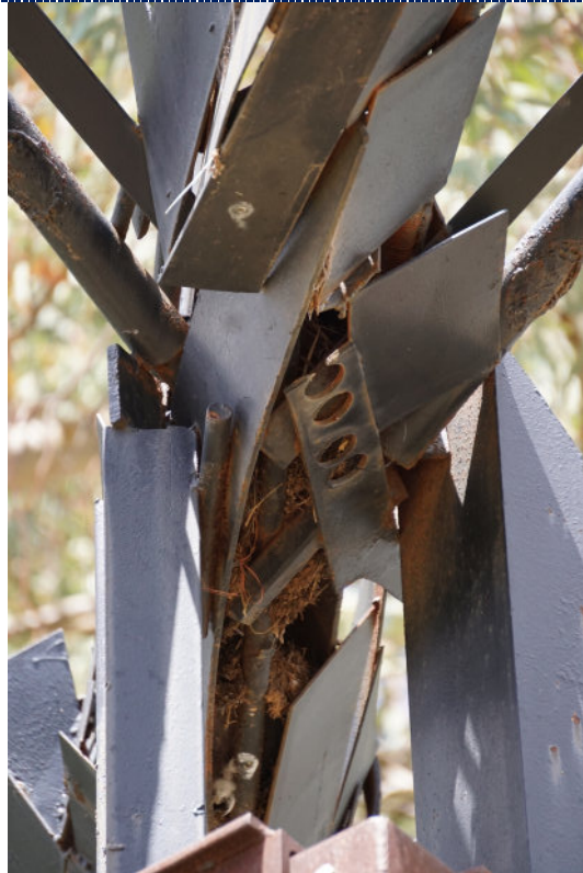
Figure 14: Detail – paint loss and corrosion to iron substrate; accumulated biomatter and spider webs within.
