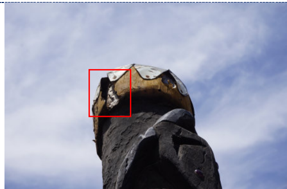
Figure 36: Detail – Pole 5, exterior, UV degradation (darkening) to wood surface, large loss to wood on exterior side of the pole's (top of pole, highlighted in red).
