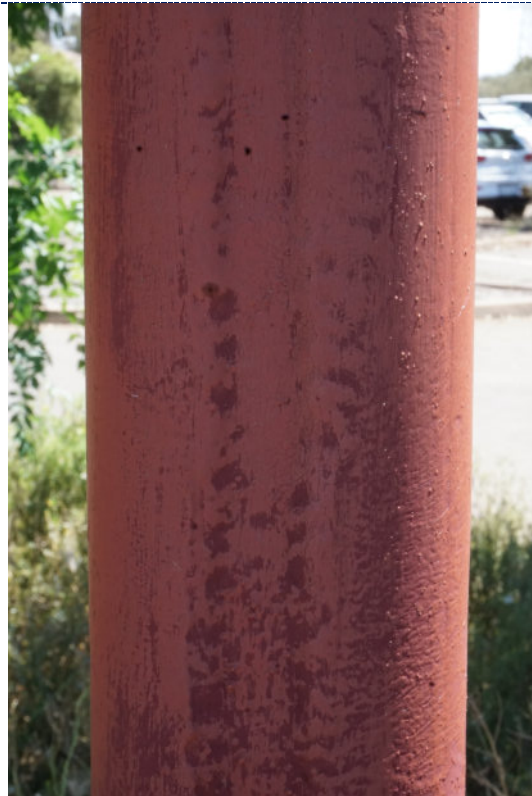
Figure 10: Detail – flaking paint loss with overpaint.
