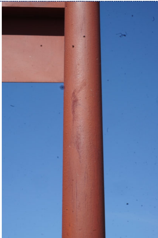
Figure 7: Detail – paint chalking, overpaint.
