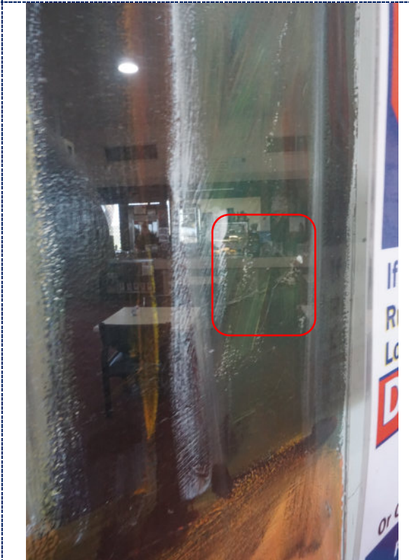
Figure 5: Section 1 – Detail – surface cracks with loss.
