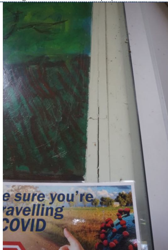
Figure 4: Section 1 – surface cracks.
