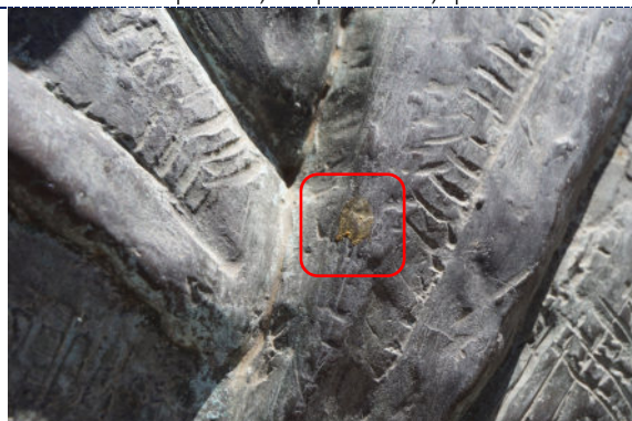
Figure 13: Detail – atmospheric pollution-driven copper corrosion product and bird excrement.
