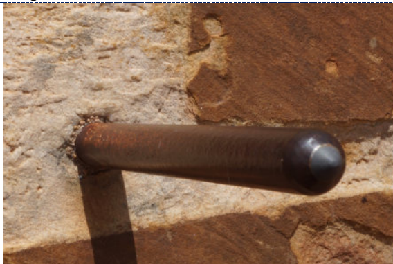
Figure 7: Details – verso, upper center, protruding armature with stable oxidation layer.
