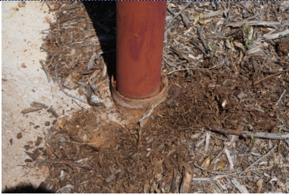
Figure 5: Detail – accumulation of biomatter at base; corrosion to iron.
