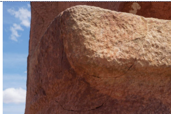
Figure 18: Detail – base, lower corner underside, cracks.
