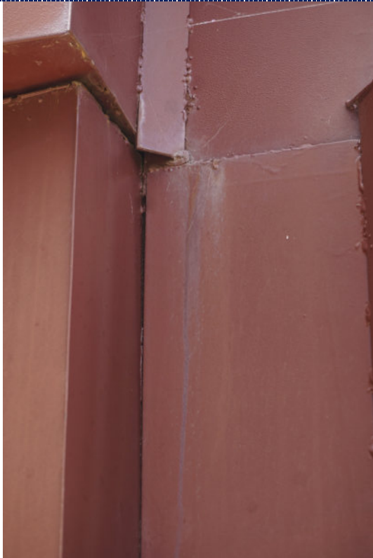
Figure 17: Detail – paint fading and degradation; dirt particulate and spider webs.
