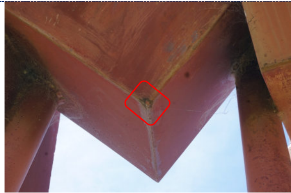
Figure 12: paint chalking, flaking paint loss with overpaint; dirt particulate and spider webs; surface corrosion at corner (circle).
