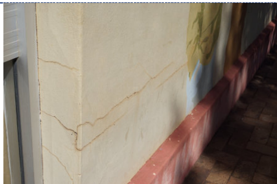
Figure 9: Detail – surface cracks and deformation to the mortar; chalking (UV degradation) and fading of the paint; staining to the exterior of the cracks.
