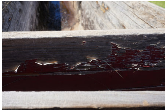
Figure 21: Detail – exterior, degraded and peeling maroon paint, UV degradation (darkening) to wood surface.
