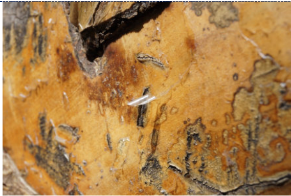
Figure 9: Detail – exterior, degraded and peeling varnish, UV degradation (darkening) to wood surface.
