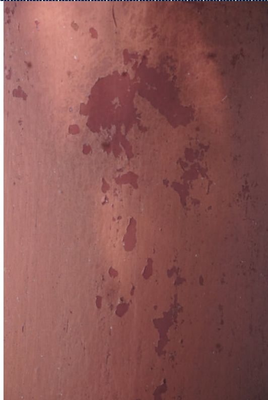
Figure 8: Detail – flaking paint loss; paint chalking. The two shades of red paint suggest the surface was repainted.
