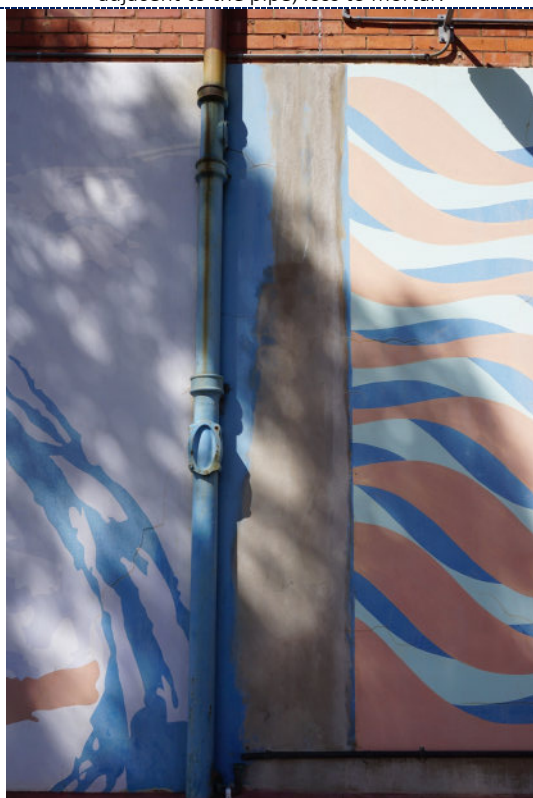
Figure 15: Detail – surface cracks and deformation to the mortar; chalking (UV degradation) and fading of the paint; staining to the exterior of the cracks; large loss to the paint adjacent to the pipe.
