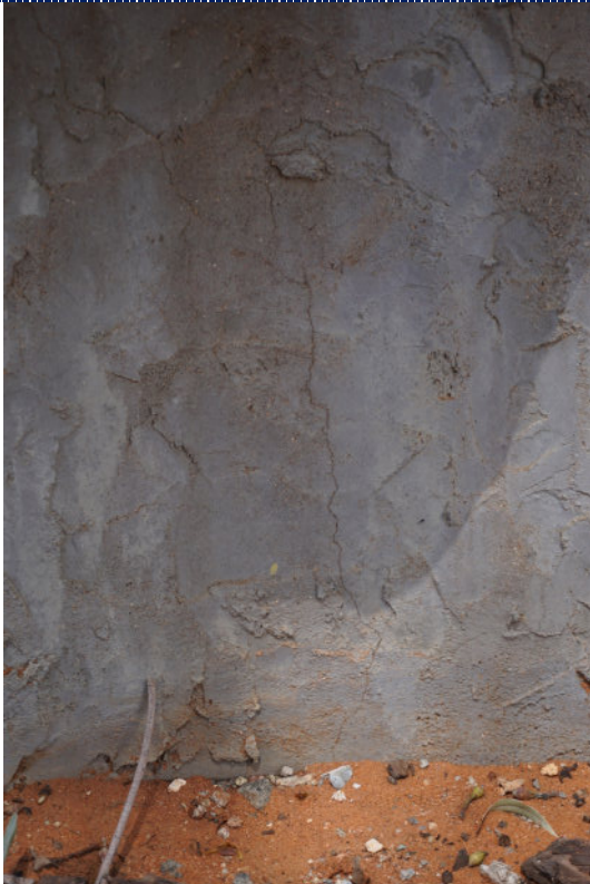
Figure 35: Figure 3 – Detail – dirt particulate, surface cracks.
