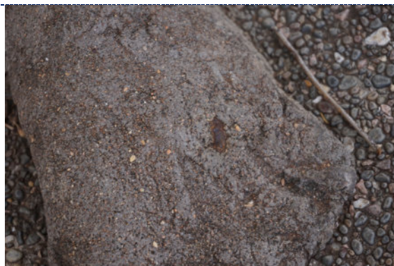
Figure 6: Figure 1 – Detail – dirt particulate, small loss revealing internal iron armature.
