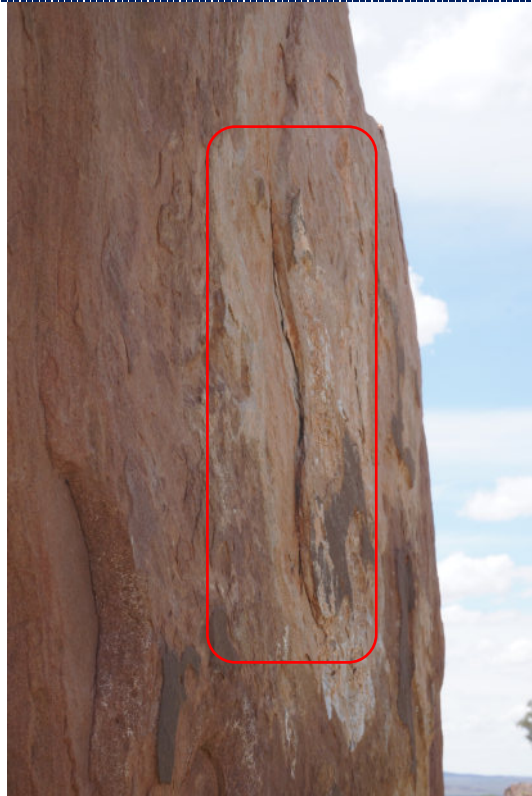
Figure 14: Detail – possible evidence of surface delamination.
