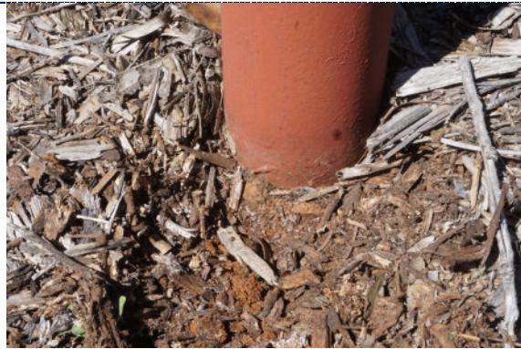
Figure 5: Detail – accumulation of biomatter at base.
