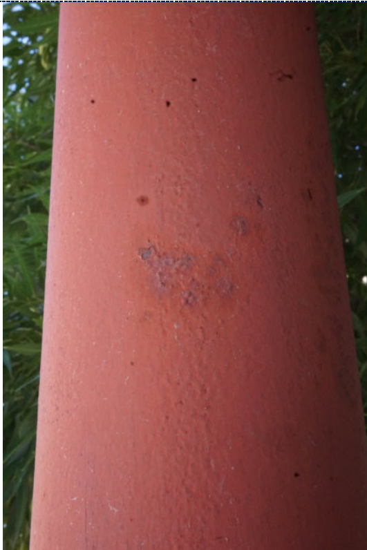
Figure 7: Detail – paint chalking, flaking paint loss with corrosion.
