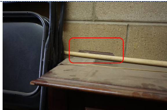
Figure 8: Detail – separated wooden component in figure 6.
