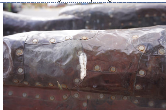
Figure 6: Detail – exterior, zinc nail heads; bird excrement.
