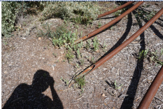
Figure 7: Detail – dirt particulate; rolled steel mounted at ground; accumulation of biomatter.
