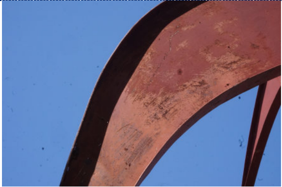
Figure 6: Detail – chalking paint, flaking paint loss, abrasions and corrosion; overpaint.
