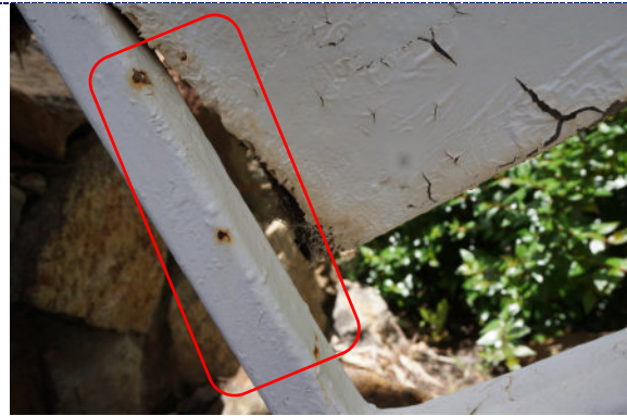
Figure 16: Detail – small areas of iron corrosion products at base.
