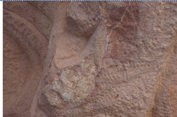
Figure 10: Detail – minor stone delamination.
