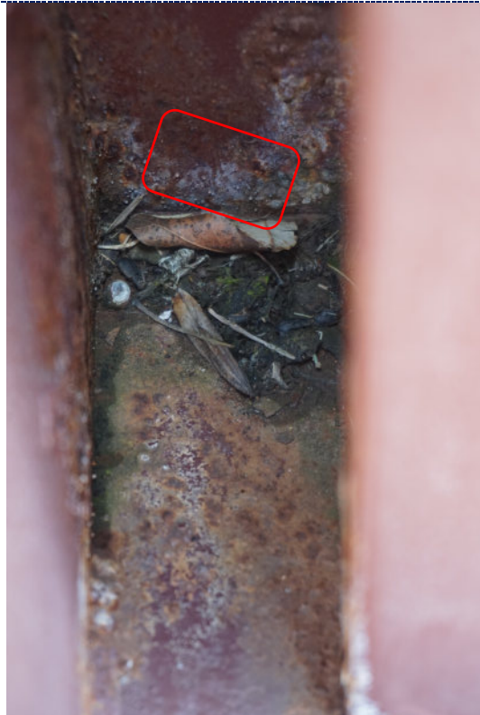
Figure 20: Detail – paint loss and corrosion to iron substrate; accumulation of dirt particulate.
