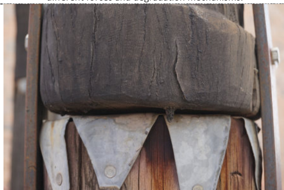
Figure 93: Detail – Pole #2003.0023, Untitled , exterior, exterior, UV degradation (darkening) to wood surface throughout. Tarnishing and iron corrosion noted on metal components and fastenings.
