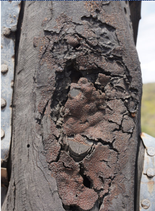
Figure 15: Detail – Pole 2, exterior, UV degradation (darkening) to wood surface, significant cracking of wood, and build-up of sap-like accretions.
