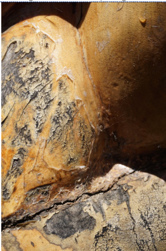
Figure 7: Detail – exterior, degraded and peeling varnish, UV degradation (darkening) to wood surface.
