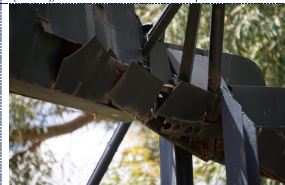
Figure 11: Detail – paint loss and corrosion to iron substrate; accumulated biomatter and spider webs within.
