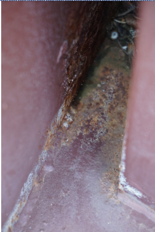
Figure 19: Detail – paint loss and corrosion to iron substrate; accumulation of dirt particulate.
