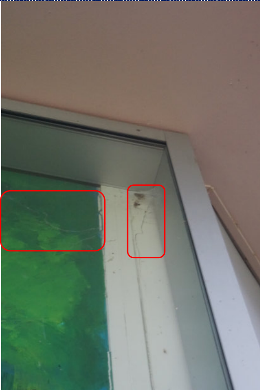
Figure 9: Section 1 – Detail – surface cracks and spider webbing.
