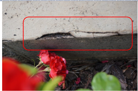
Figure 10: Detail – dirt particulate, crack and loss to plinth render.
