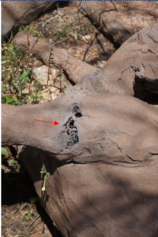
Figure 15: Detail – loss to concrete fondue revealing chicken wire and iron armature.
