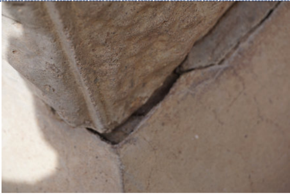
Figure 21: Detail – loss to concrete render.
