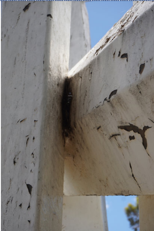
Figure 7: Detail – dirt particulate and surface paint loss and crazing.
