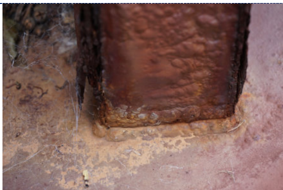
Figure 15: Detail – paint fading and degradation; corrosion to iron substrate; dirt particulate.
