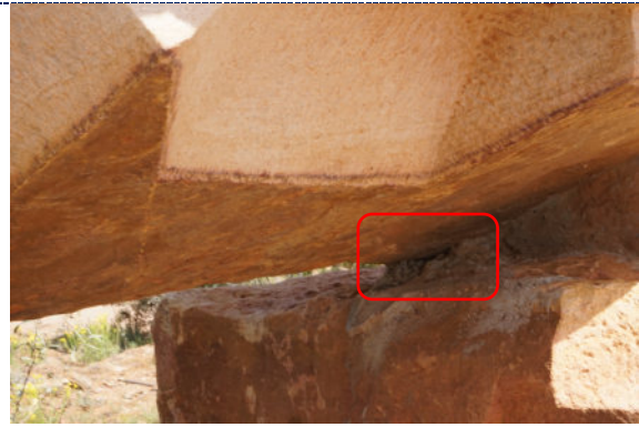
Figure 10: Detail – small gap in mortar.
