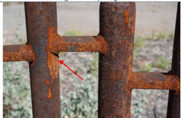
Figure 6: Detail – dirt particulate; surface flash rusting at new welds created during manufacture of artwork.
