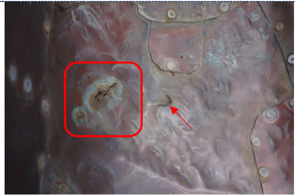
Figure 18: Detail – exterior, corrosion perforating copper plate; minor corrosion to zinc nail heads.
