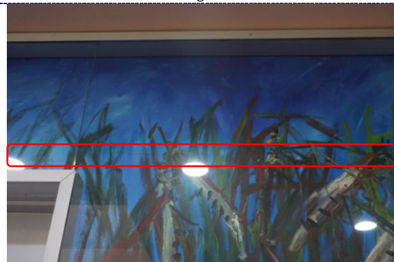
Figure 38: Section 3 – Detail – horizontal surface crack.
