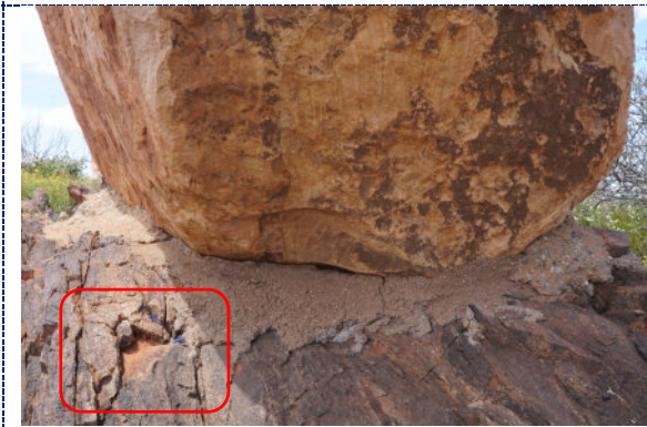
Figure 7: Detail – concrete plinth supporting sculpture with small loss to concrete.
