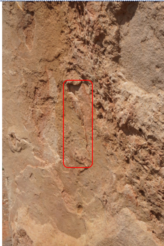
Figure 8: Detail – stone delamination and small vertical crack.
