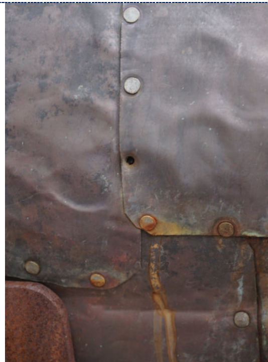
Figure 28: Detail – exterior, missing nail; corroding zinc-iron nails and iron corrosion staining.
