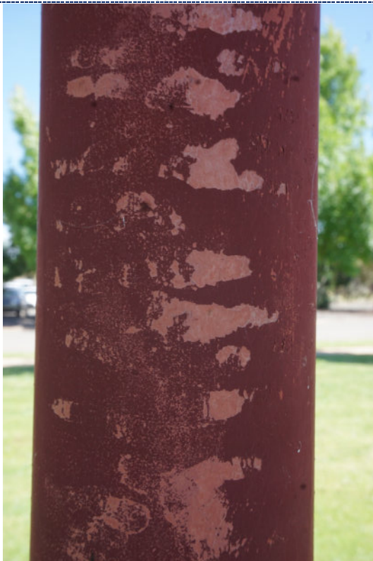
Figure 15: Detail – flaking paint and paint loss.
