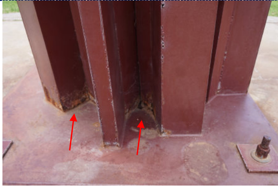
Figure 21: Detail – paint fading and degradation; dirt particulate; iron corrosion.
