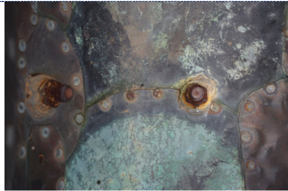
Figure 24: Detail – interior, dirt particulate, green copper corrosion in areas where water pools; corroded bolts where mounts are attached.
