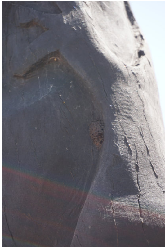
Figure 90: Detail – Pole 12, exterior, UV degradation (darkening) to wood surface, cracks and splitting following the grain of the wood, cobwebs and dirt particulate noted throughout.
