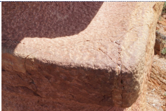
Figure 17: Detail – base, lower corner, cracks.
