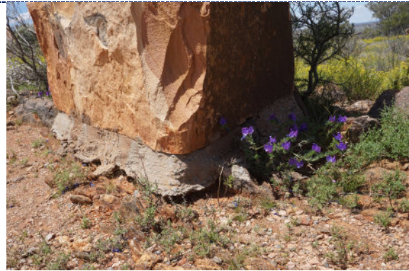
Figure 6: Detail – possible erosion to soil under concrete mortar.
