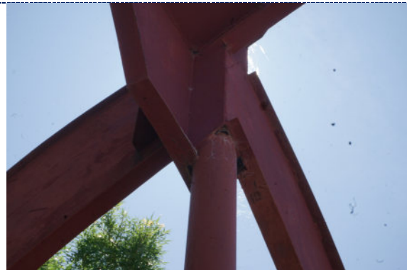
Figure 12: Detail – small holes noted at welding joint and spider webs.
