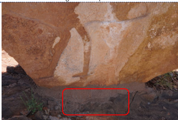
Figure 5: Detail – rear cement/concrete at base; crack in cement.
