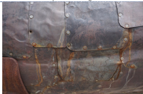
Figure 34: Detail – exterior, missing and loose nail; corroding zinc-iron nails; significant iron corrosion staining.
