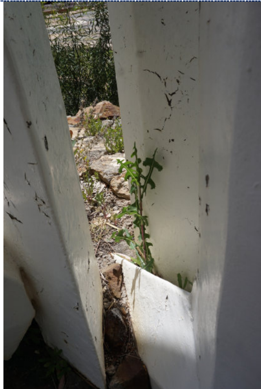
Figure 8: Detail – dirt particulate and surface paint loss and crazing; biogrowth in crevices.
