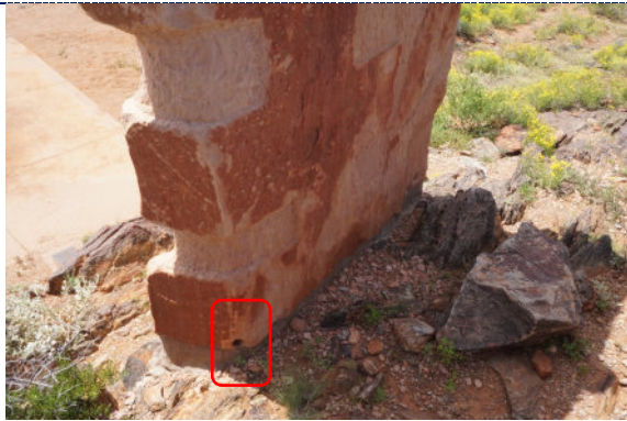
Figure 5: Detail – hole at base; minor surface abrasions.
