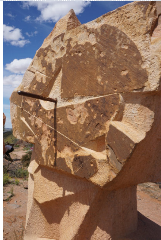
Figure 14: Details – surface abrasions and delamination.
