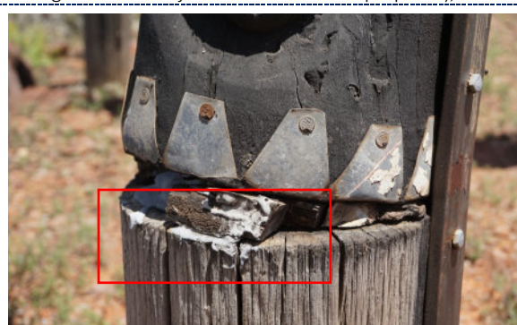
Figure 88: Detail – Pole 12, exterior, UV degradation (darkening) to wood surface, iron corrosion on metal components, including the iron nails, and a build up of loose material on the wood base suggestive of insect activity (highlighted in red).
