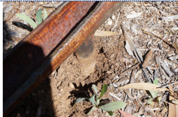
Figure 8: Detail – dirt particulate; rolled steel mounted at ground; accumulation of biomatter.
