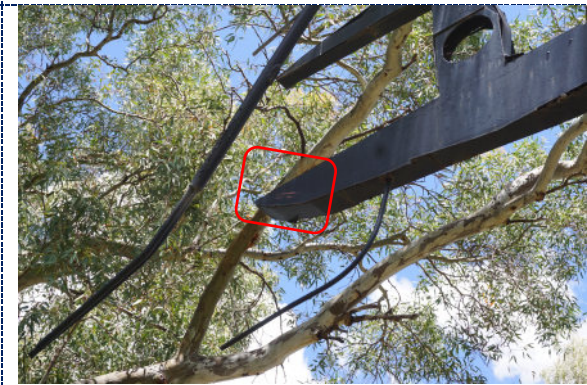
Figure 5: Detail – paint loss and corrosion to iron substrate.
