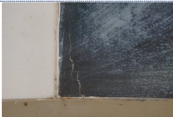
Figure 25: Section 2 – Detail – surface cracks.
