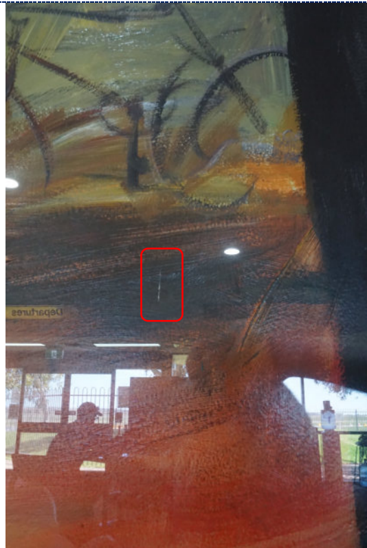
Figure 6: Section 1 – Detail – white surface accretion.
