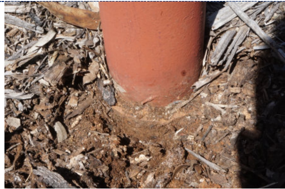
Figure 6: Detail – accumulation of biomatter at base; corrosion to iron.
