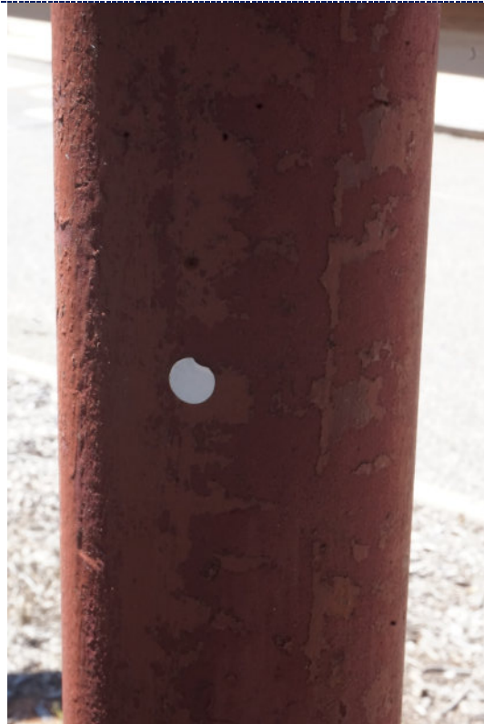
Figure 8: Detail – paint chalking, flaking, overpaint; white sticker accretion.
