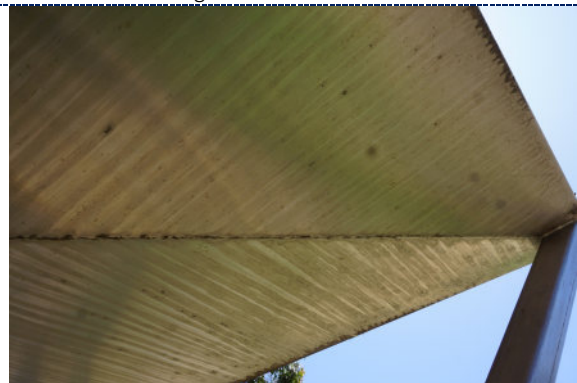
Figure 12: Detail – dirt particulate accumulation along the bottom diamond edges and water streaks.
