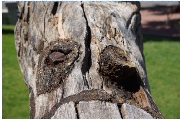
Figure 20: Detail – exterior, corroded iron bolts and peeling varnish. A tar-like accretion is evident within a joint and around the iron bolts.
