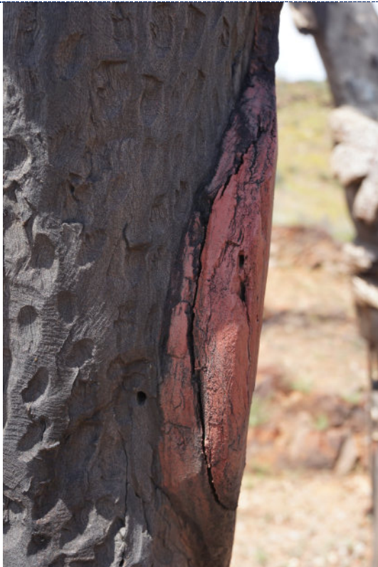
Figure 41: Detail – Pole 6, exterior, UV degradation (darkening) to wood surface, extensive cracking, and losses to raised carved wood designs and associated paint losses likely due UV degradation and full exposure to the elements.
