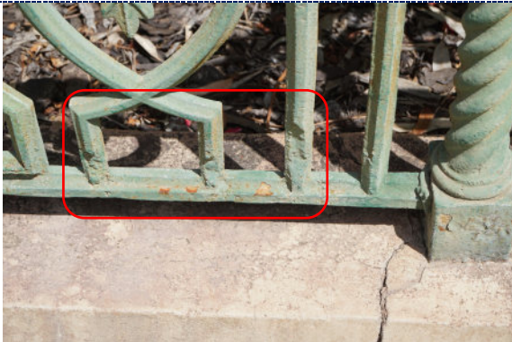
Figure 25: Detail – cracks to plinth render; loss and degradation of green paint on cast iron fencing; iron corrosion product; losses to iron, previously repaired.
