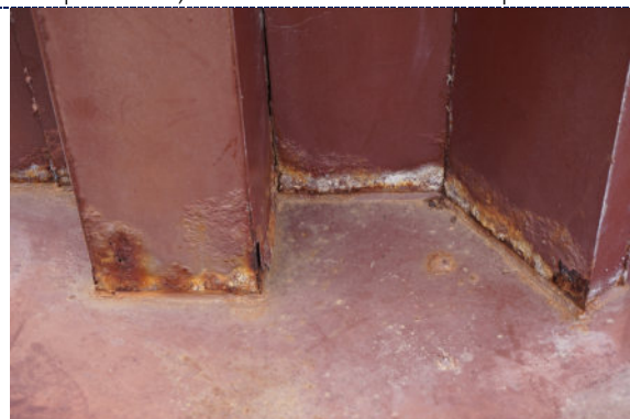
Figure 16: Detail – paint fading and degradation; dirt particulate and surface accretions (white); iron corrosion.
