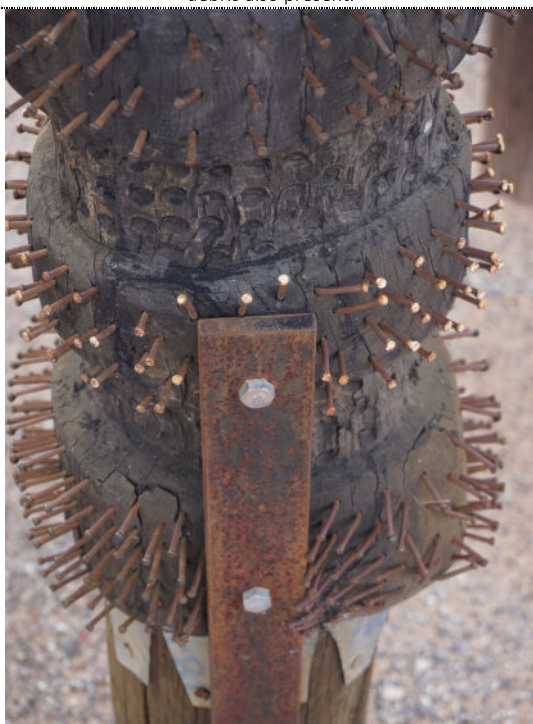
Figure 17: Detail – Pole #2003.0017 Reconciliation , exterior, corroded iron nails and metal structural components, UV degradation (darkening) to wood surface, and fine cracks along the grain of the wood.
