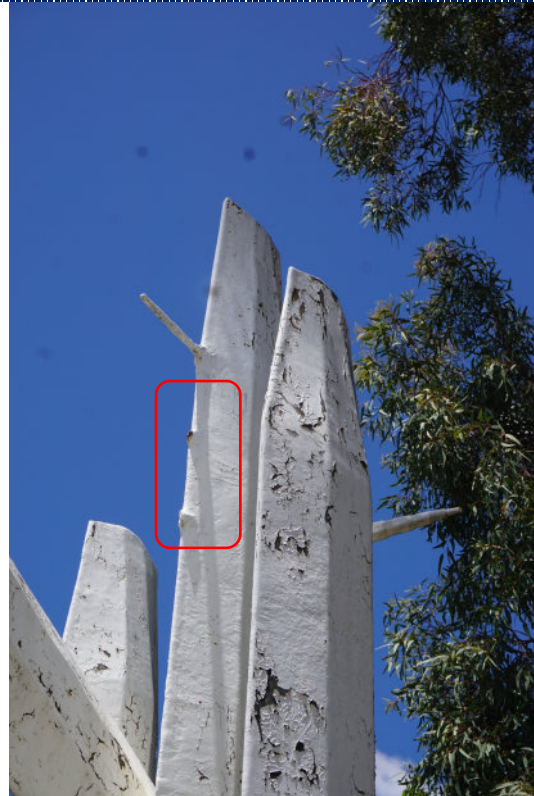
Figure 18: Detail – dirt particulate and significant surface paint loss and crazing; missing spikes.
