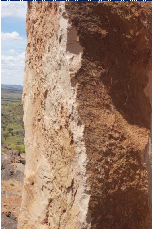
Figure 9: Detail – minor stone delamination.
