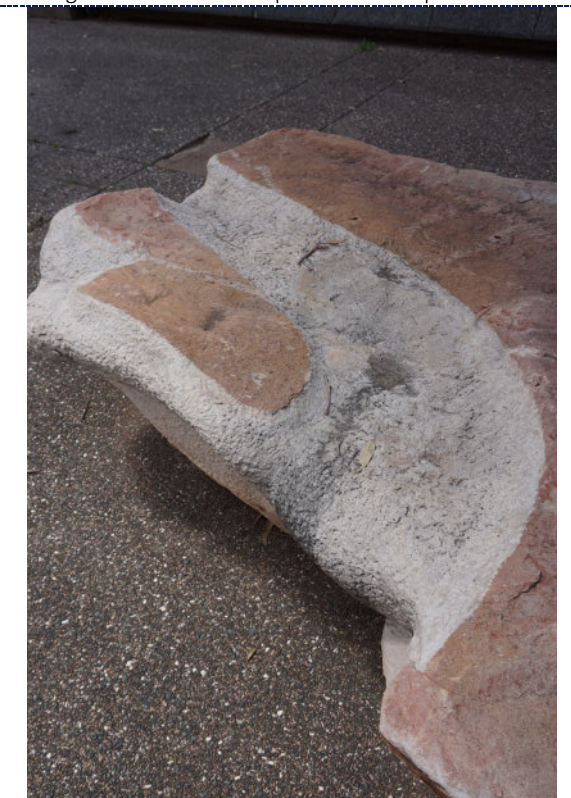
Figure 30: Detail – Component 4 – dirt particulate from water pooling.
