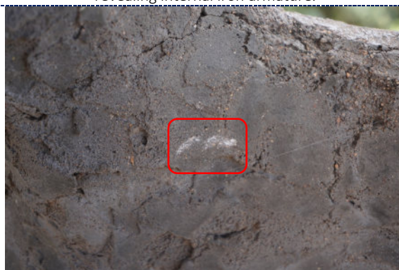
Figure 8: Figure 1 – Detail – dirt particulate, surface cracks and surface abrasion.
