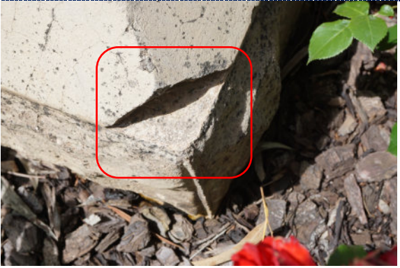
Figure 16: Detail – small cracks and loss to plinth render.
