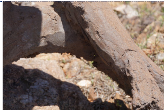
Figure 18: Detail – horizontal crack.
