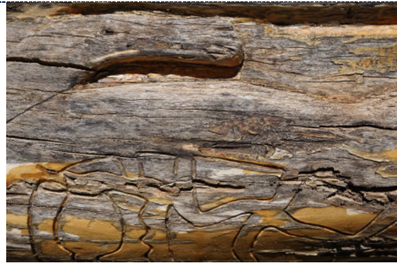
Figure 10: exterior, degraded and peeling varnish, UV degradation (darkening) to wood surface.
