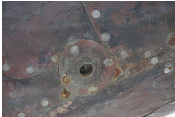
Figure 29: Detail – exterior, dirt particulate, spider webs; corrosion to zinc nail heads; biomatter clogging drains.
