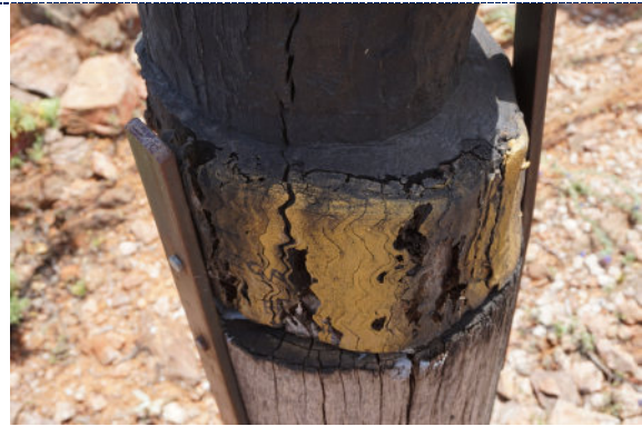
Figure 28: Detail – Pole 4, exterior, UV degradation (darkening) to wood surface, losses to wood likely associated with past insect activity, iron corrosion on metal support brackets.
