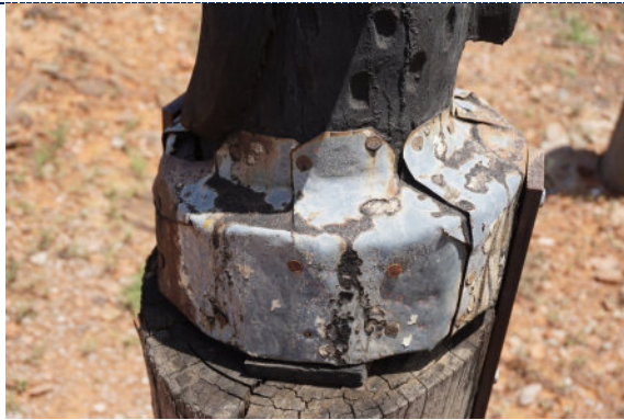
Figure 33: Detail – Pole 5, exterior, UV degradation (darkening) to wood surface, degradation of metal and presence of iron corrosion products. Dirt particulate is present throughout.
