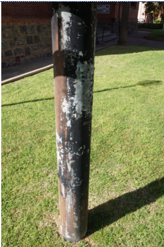
Figure 7: Detail – support pole. Extensive loss of paint layer exposing steel substrate. Surface corrosion occurring.
