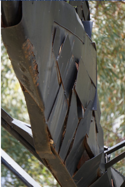
Figure 13: Detail – paint loss and corrosion to iron substrate; accumulated biomatter and spider webs within.
