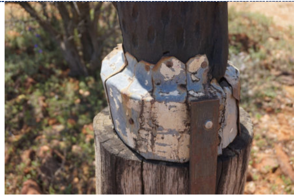
Figure 48: Detail - Pole 7, exterior, UV degradation (darkening) to wood surface, chemical degradation of the spherical metal components, including the presence of pitting and iron corrosion products on the iron nails.
