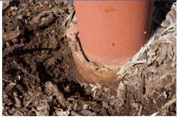
Figure 12: Detail – accumulation of biomatter at base; corrosion to iron.
