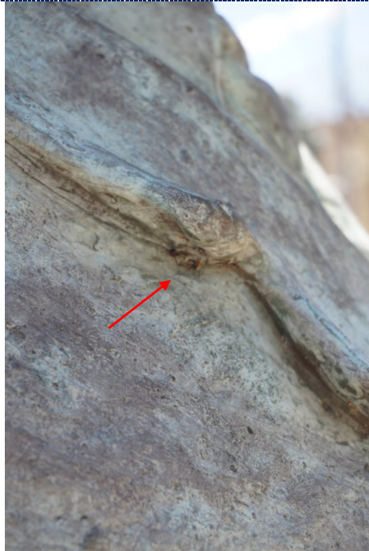
Figure 14: Detail – atmospheric pollution-driven copper corrosion product, dirt particulate, spider webs.
