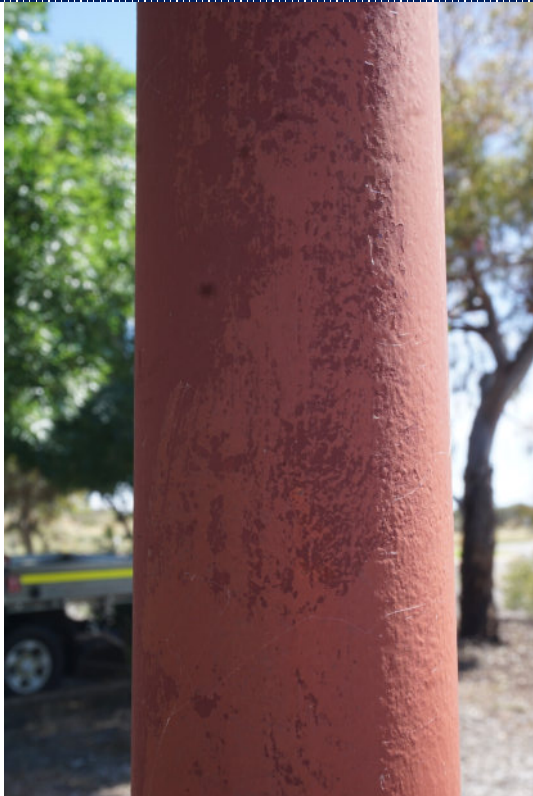
Figure 8: Detail – paint chalking, flaking paint loss with overpaint.
