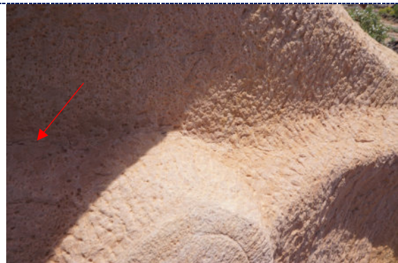
Figure 10: Detail – horizontal crack with minor stone delamination.
