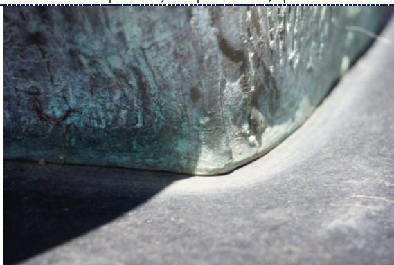
Figure 13: Detail – atmospheric pollution-driven copper corrosion product, dirt particulate, spider webs.
