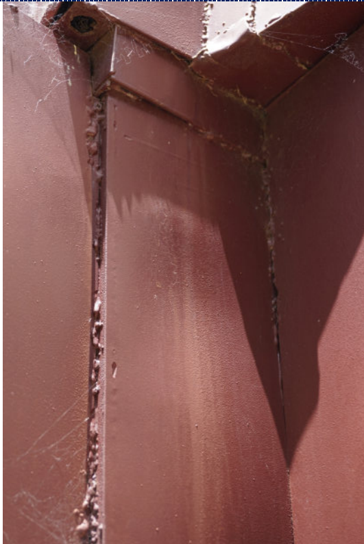
Figure 11: Detail – paint fading and degradation; dirt particulate and spider webs.
