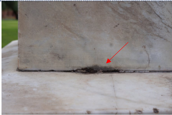
Figure 9: Detail – dirt particulate, pointing loss at join.
