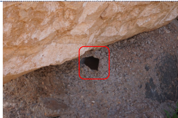
Figure 6: Detail – hole in concrete base.
