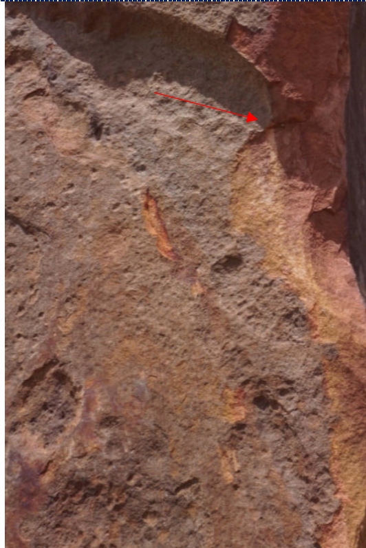
Figure 20: Detail – Surface delamination.
