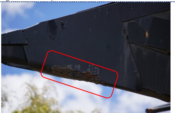
Figure 10: Detail – paint loss and corrosion to iron substrate.
