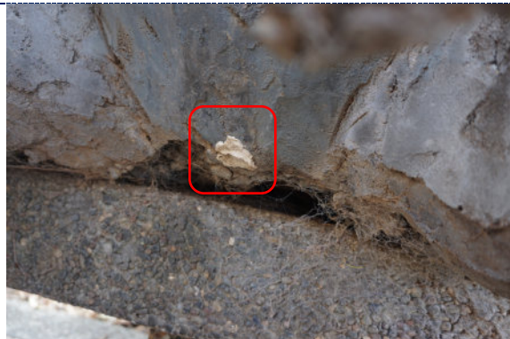
Figure 33: Figure 3 – Detail – dirt particulate, surface cracks and spider webs.
