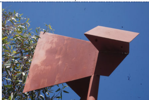
Figure 9: Detail – paint chalking, flaking paint loss with overpaint;
