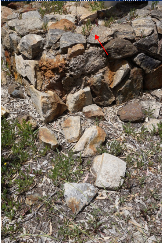
Figure 5: Detail – stones separated from the plinth; biogrowth in crevices (arrow).
