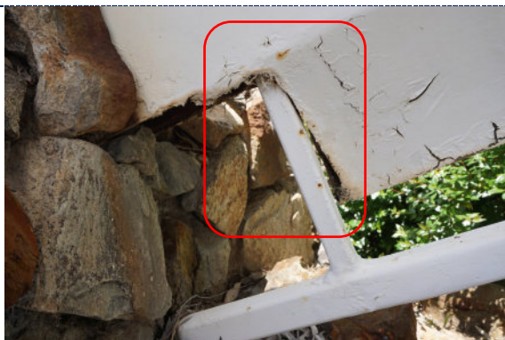
Figure 13: Detail – small areas of iron corrosion products at base.
