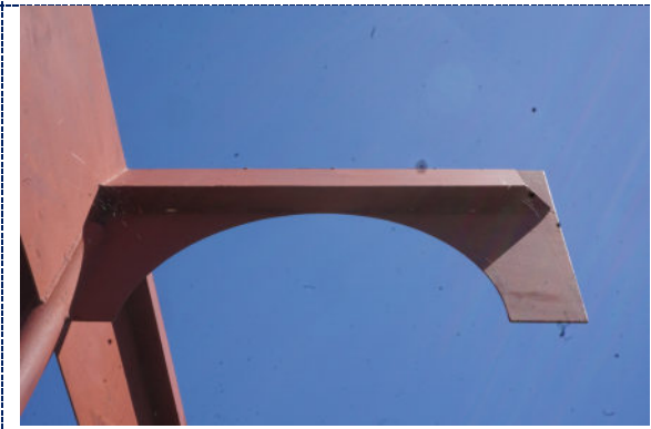
Figure 11: Detail – paint chalking, overpaint.
