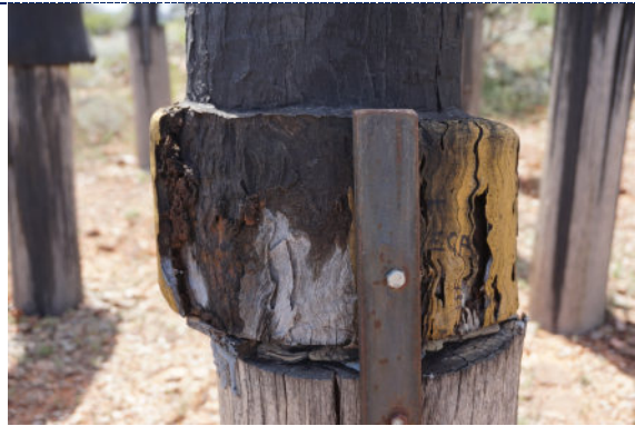
Figure 27: Detail – Pole 4, exterior, UV degradation (darkening) to wood surface, losses to wood likely associated with past insect activity, iron corrosion on metal support brackets. Dirt particulate is present throughout.
