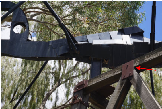
Figure 15: Detail – surface oxidation layer on structural brackets (arrow); UV and water weathering to wooden frame.
