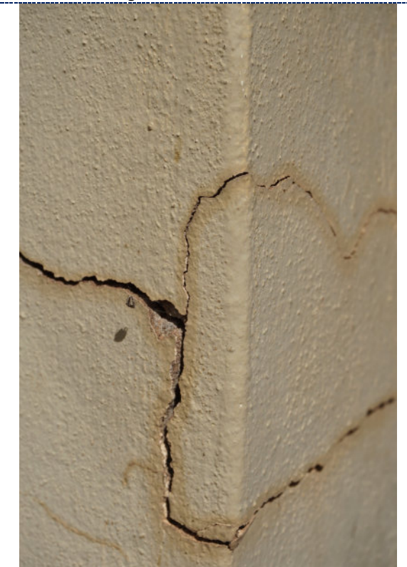
Figure 11: Detail – surface cracks and deformation to the mortar; chalking (UV degradation) and fading of the paint; staining to the exterior of the cracks; small losses.
