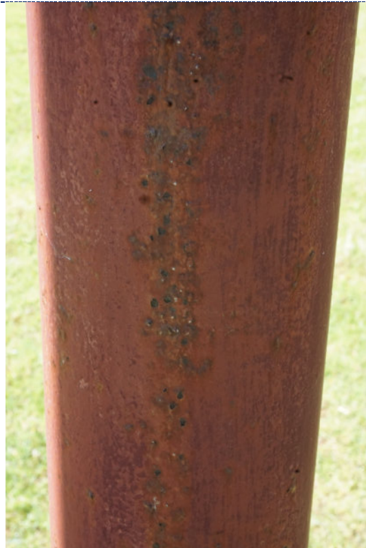
Figure 14: Detail – paint chalking, flaking paint loss with overpaint; corrosion in areas of paint loss.
