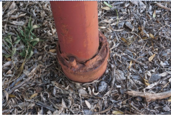
Figure 5: Detail – base plinth, paint chalking, flaking paint loss with corrosion and putty deterioration.
