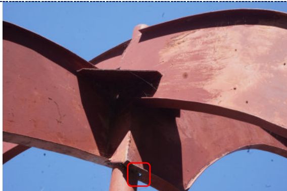
Figure 13: Detail – chalking paint, flaking paint loss, abrasions and corrosion; overpaint; corrosion resulting in perforation of the substrate (small hole).
