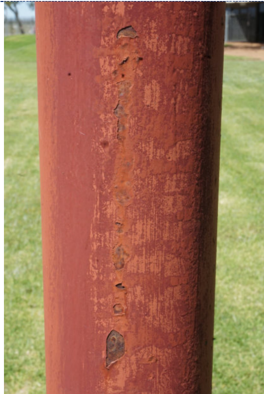
Figure 8: Detail – paint chalking, flaking paint loss with overpaint; corrosion in areas of paint loss.
