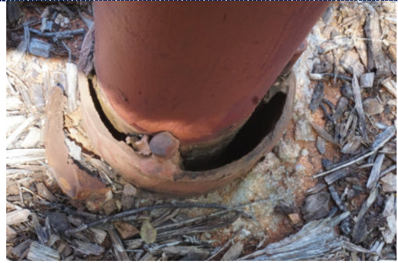
Figure 16: Detail – deteriorated putty with loss throughout base plinth; ingress of water possible, leading to corrosion.
