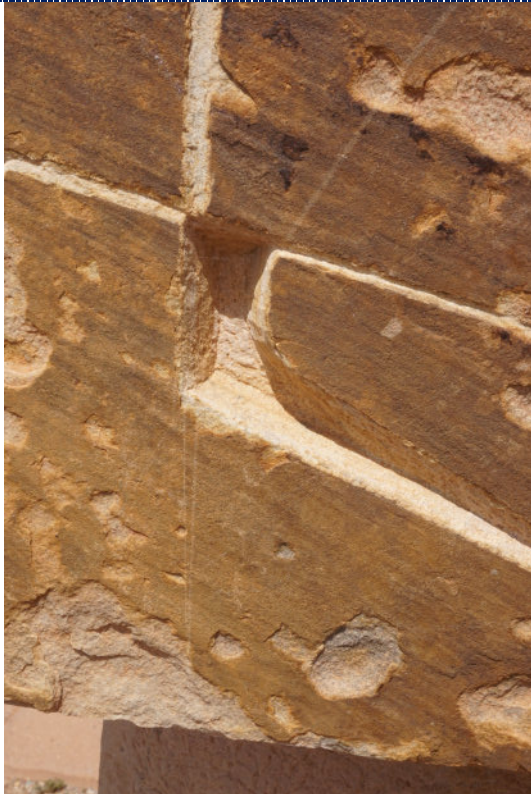
Figure 5: Details – surface abrasions and delamination.
