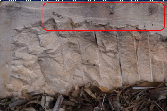
Figure 16: Detail – Component 2 – dirt particulate and bird excrement.
