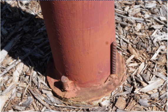
Figure 6: Detail – paint chalking, flaking paint loss with overpaint; corrosion at base.
