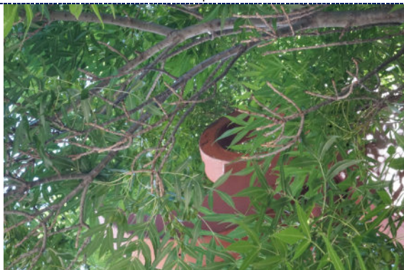
Figure 13: Detail – tree foliage intrusion, risks staining and warping of structure.
