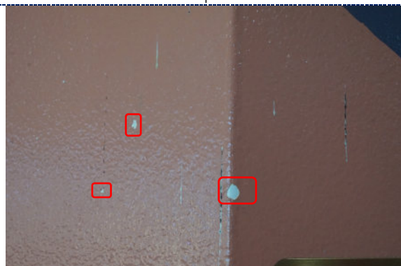
Figure 34: Work 9 – Detail below – 3 x losses with multiple surface accretions.
