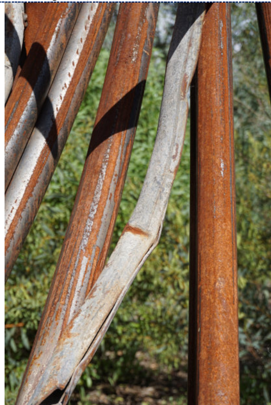
Figure 10: Detail – dirt particulate; surface corrosion.
