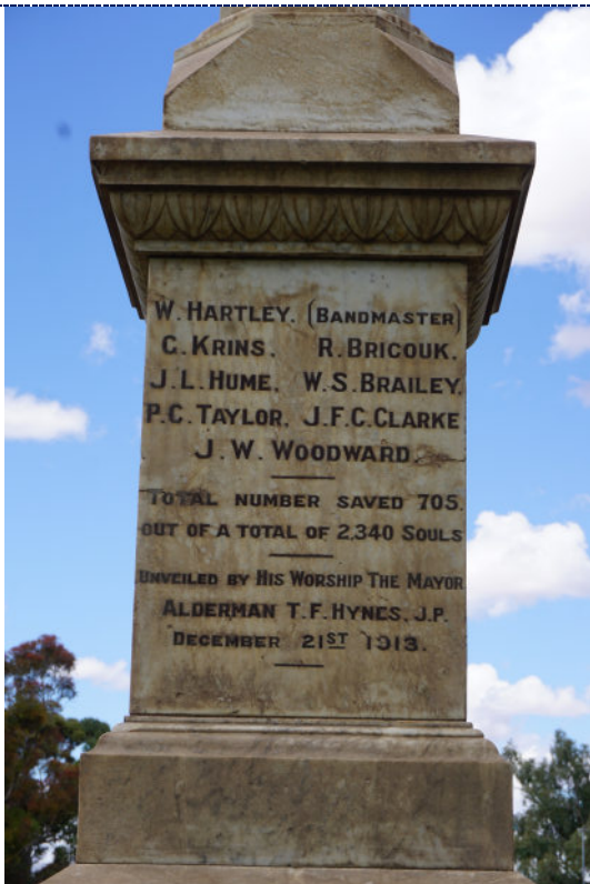
Figure 7: Detail – back, dirt particulate and stone discolouration.
