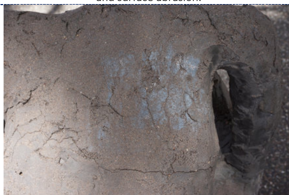
Figure 10: Figure 1 – Detail – dirt particulate, surface cracks and surface paint (likely graffiti).
