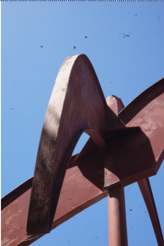
Figure 7: Detail – chalking paint, flaking paint loss, abrasions and corrosion; overpaint.
