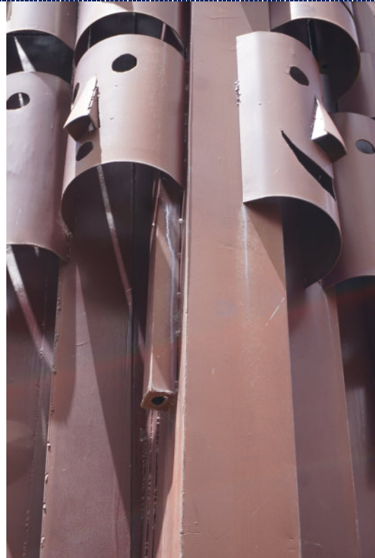
Figure 12: Detail – paint fading and degradation; dirt particulate and spider webs.
