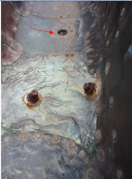
Figure 19: Detail – interior, dirt particulate, green copper corrosion in areas where water pools; corroded bolts where mounts are attached; biomatter clogging drains.
