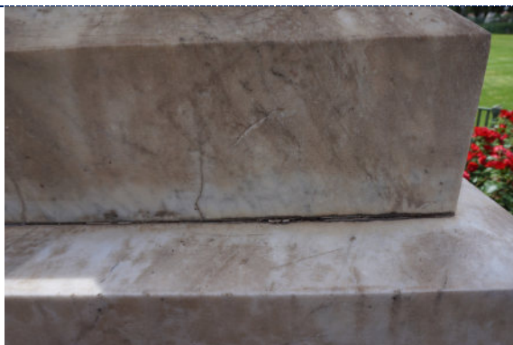
Figure 13: Detail – dirt particulate, small vertical crack in marble substrate; small losses to mortar pointing.
