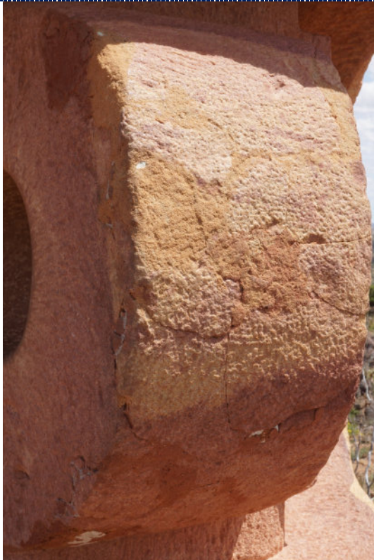
Figure 6: Detail – previous repair.
