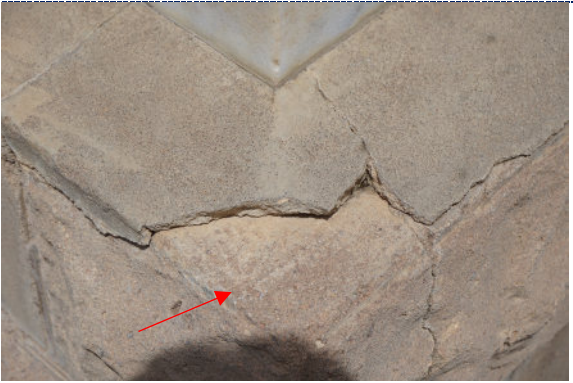
Figure 20: Detail – small cracks and loss to plinth render.
