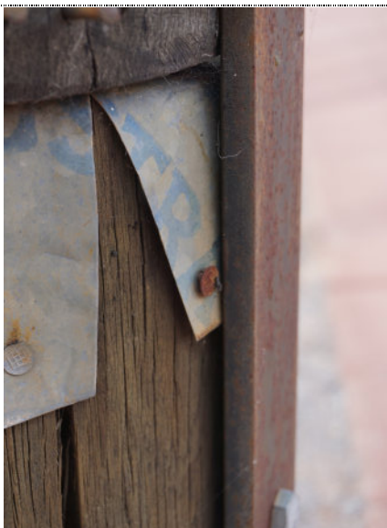
Figure 13: Detail – Pole #2003.0017 Reconciliation , exterior, corroded iron nails and metal components, UV degradation (darkening) to wood surface, and fine cracks along the grain of the wood.
