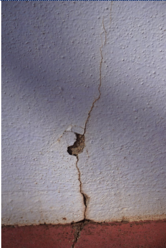
Figure 17: Detail – surface cracks and deformation to the mortar; chalking (UV degradation) and fading of the paint; staining to the exterior of the cracks; small losses.
