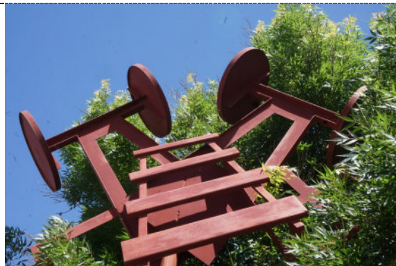
Figure 15: Detail – paint chalking, flaking, overpaint.
