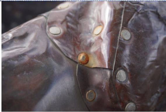
Figure 11: Detail – exterior, corroding zinc-plated nail.
