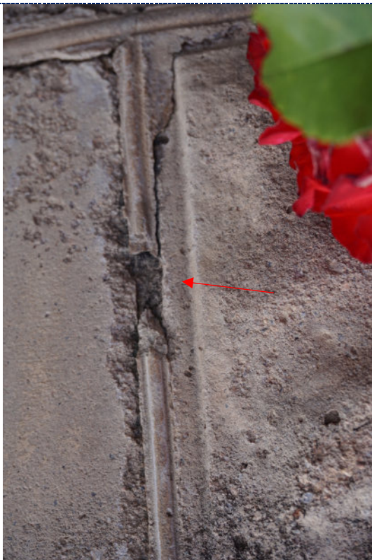
Figure 11: Detail – crack and loss to plinth concrete pointing.
