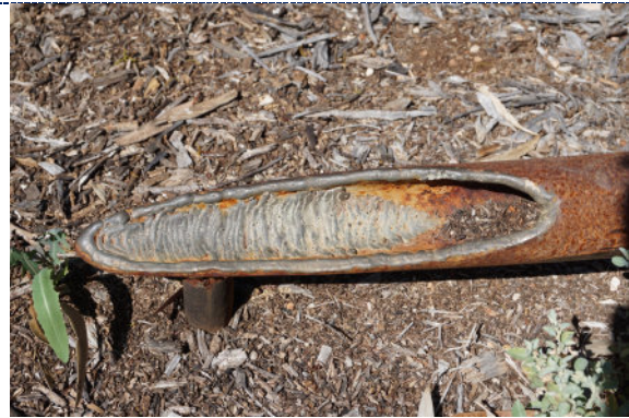
Figure 6: Detail – dirt particulate within tube; surface corrosion.
