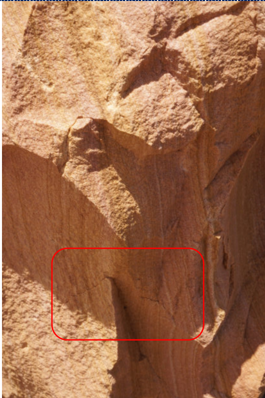
Figure 13: Detail – small crack and possible delamination present.
