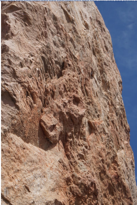
Figure 7: Detail – minor stone delamination.
