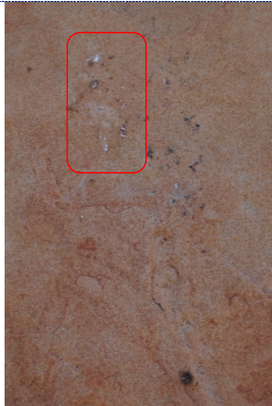
Figure 8: Detail – white surface accretion, possibly remnants of bird excrement.
