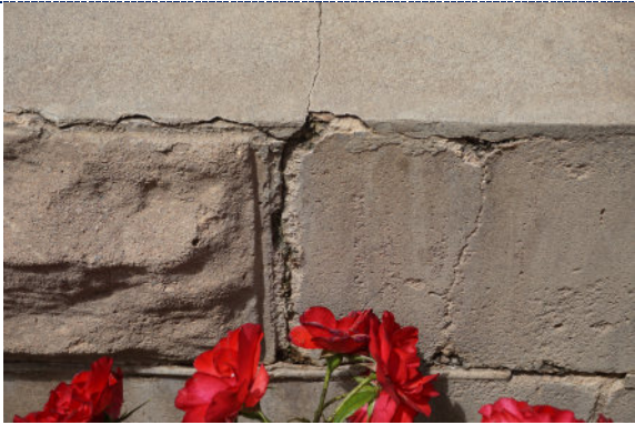
Figure 19: Detail – cracks and small losses to concrete render.
