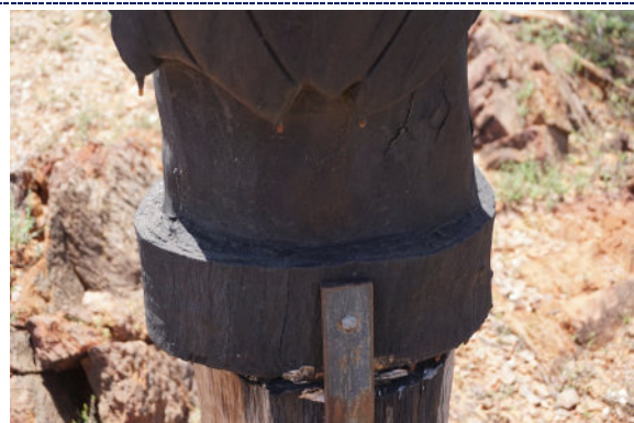
Detail 84: Detail – Pole 11, exterior, UV degradation (darkening) to wood surface, sap-like deposits (accretions) (highlighted in red). Iron corrosion products present on metal components, including the iron nails.
