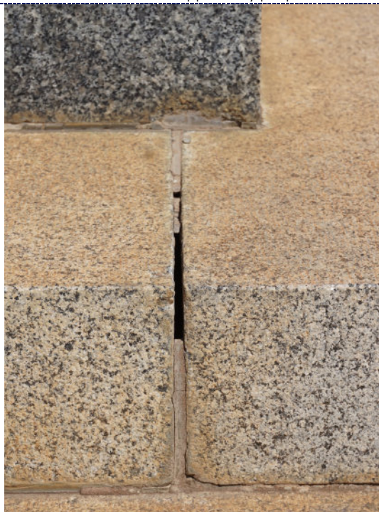
Figure 13: Detail – dirt particulate, red staining (possibly iron corrosion product) and loss to mortar pointing.
