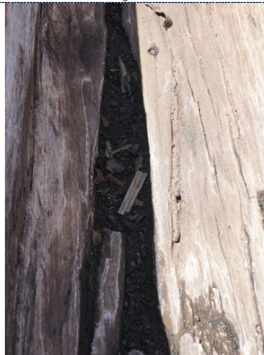
Figure 14: Detail – interior, degraded and peeling varnish, UV degradation (darkening) to wood surface. Interior poly propylene liner, silicon sealant and iron staples heavily degraded. Loose dirt particulate and debris.
