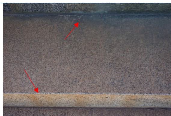
Figure 12: Detail – dirt particulate and copper corrosion product staining to granite stone; red staining at bottom may stem from iron corrosion elsewhere on the object.
