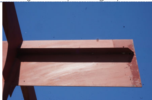
Figure 10: Detail – paint chalking, overpaint.
