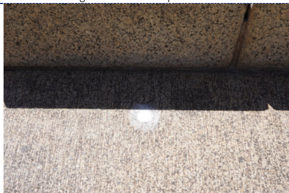
Figure 19: Detail – loss to mortar pointing and bird excrement.
