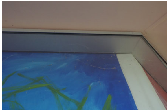
Figure 44: Section 3 – Detail – dirt particulates and spider webs.
