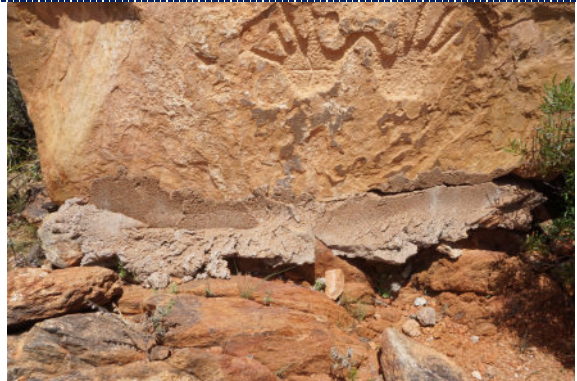
Figure 8: Detail – possible erosion to soil under concrete mortar.
