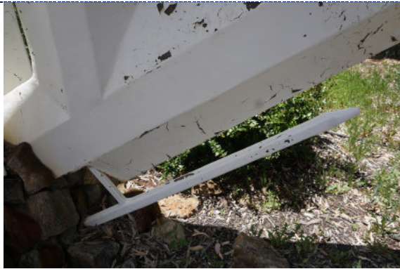
Figure 15: Detail – dirt particulate and significant surface paint loss and crazing.
