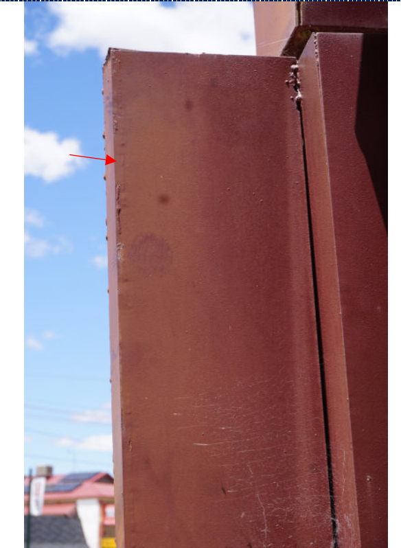
Figure 7: Detail – paint fading and degradation; dirt particulate and spider webs.
