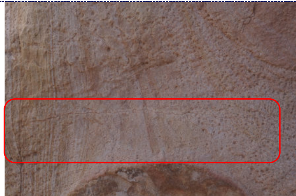
Figure 8: Detail – crack visible through centre.
