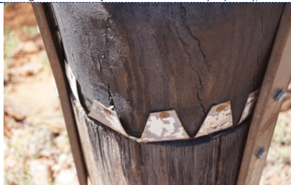
Figure 87: Detail – Pole 12, exterior, UV degradation (darkening) to wood surface, iron corrosion on metal components, including the iron nails.
