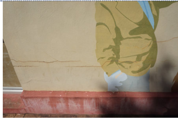
Figure 8: Detail – surface cracks and deformation to the mortar; chalking (UV degradation) and fading of the paint; staining to the exterior of the cracks.
