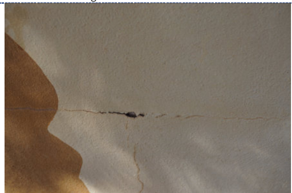
Figure 6: Detail – surface cracks and deformation to the mortar; chalking (UV degradation) and fading of the paint; staining to the exterior of the cracks; small losses.
