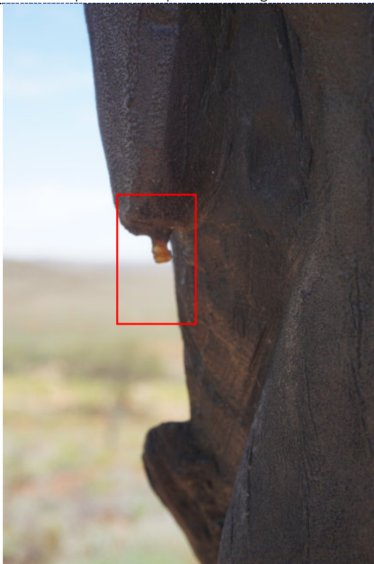
Detail 49: Detail – Pole 7, exterior, UV degradation (darkening) to wood surface, sap-like deposits (accretions) along the lower edge of the pole (highlighted in red).
