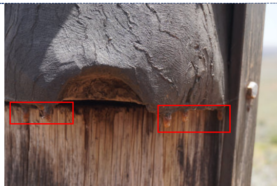
Figure 20: Detail – Pole 3, exterior, UV degradation (darkening) to wood surface, sap-like deposits (accretions) along the lower edge of the pole (highlighted in red).
