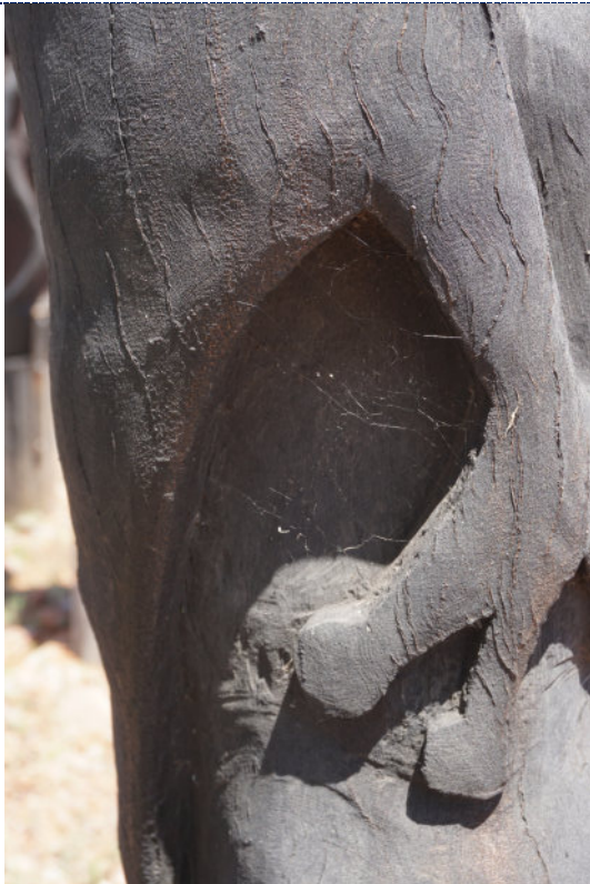
Figure 89: Detail – Pole 12, exterior, UV degradation (darkening) to wood surface, cracks and splitting following the grain of the wood, cobwebs and dirt particulate noted throughout.
