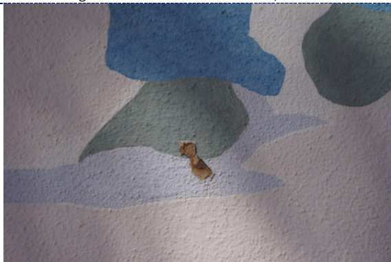
Figure 19: Detail – surface accretion; chalking (UV degradation) and fading of the paint.
