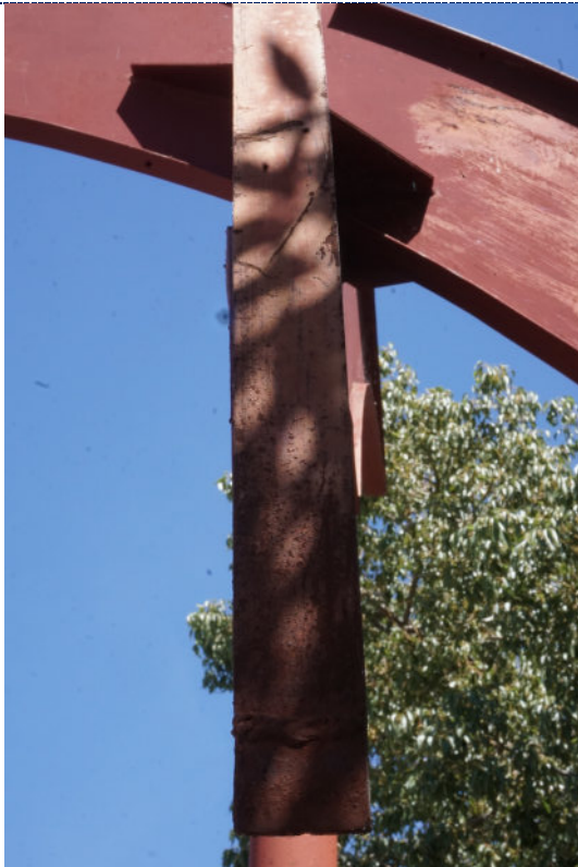
Figure 9: Detail – chalking paint, flaking paint loss, abrasions and corrosion; overpaint.
