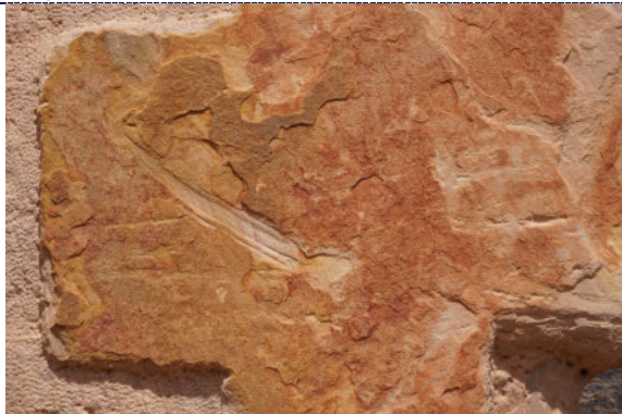
Figure 7: Detail – possible surface delamination.
