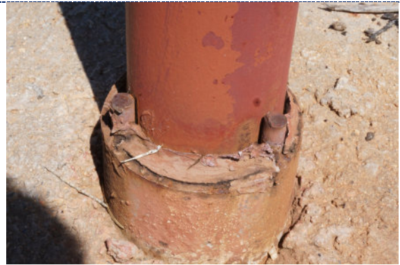
Figure 6: Detail – paint chalking, flaking paint loss with overpaint; corrosion in areas of paint loss; previous repairs (putty/silicone at base).
