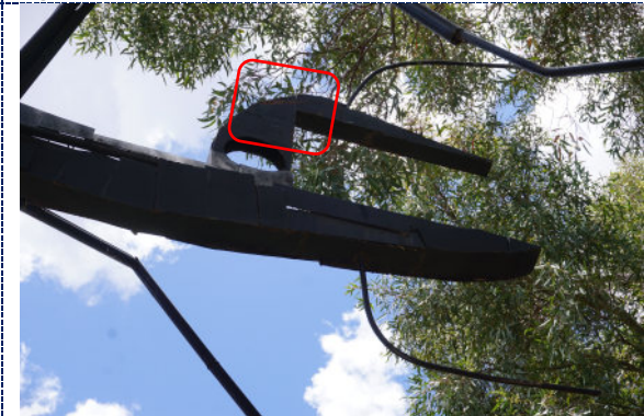
Figure 7: Detail – paint loss and corrosion to iron substrate.
