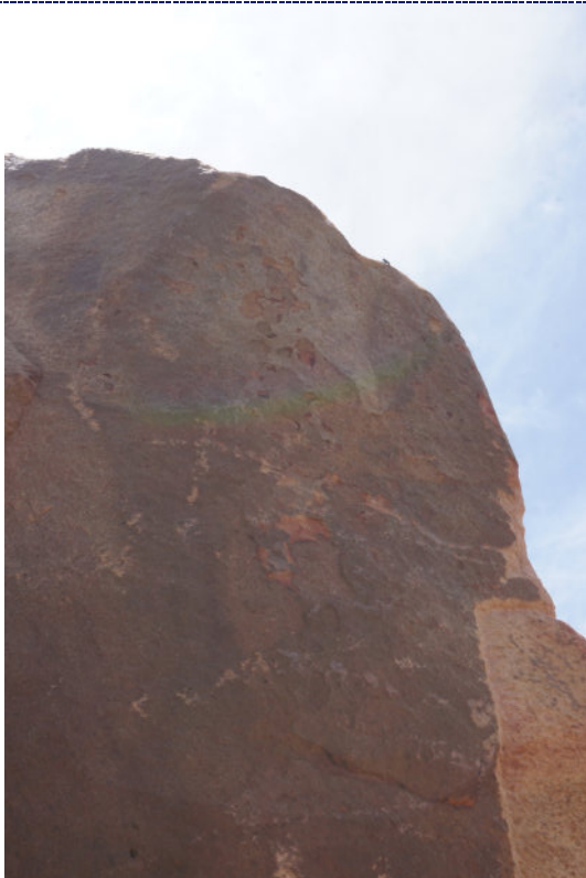
Figure 21: Detail – surface delamination.
