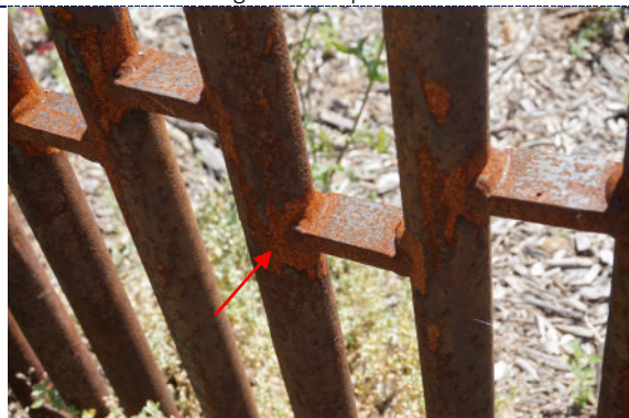
Figure 5: Detail – dirt particulate; surface flash rusting at new welds created during manufacture of artwork.
