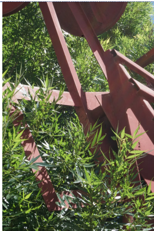
Figure 12: Detail – paint chalking, flaking, overpaint; surface corrosion; woody plant growth interaction.
