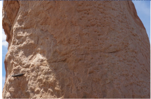
Figure 6: Detail – horizontal crack, likely occurring naturally within the stone.
