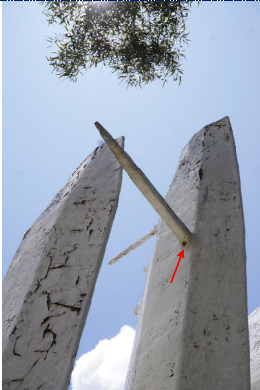
Figure 17: Detail – dirt particulate and significant surface paint loss and crazing; iron corrosion product staining (arrow).
