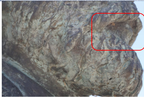
Figure 9: Detail – atmospheric pollution-driven copper corrosion product, dirt particulate, spider webs.
