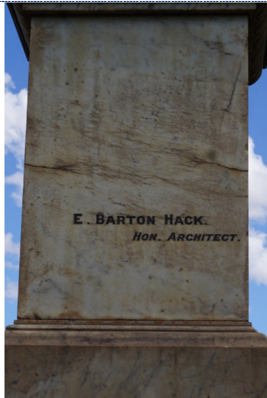
Figure 6: Detail – proper left, dirt particulate and stone discolouration.
