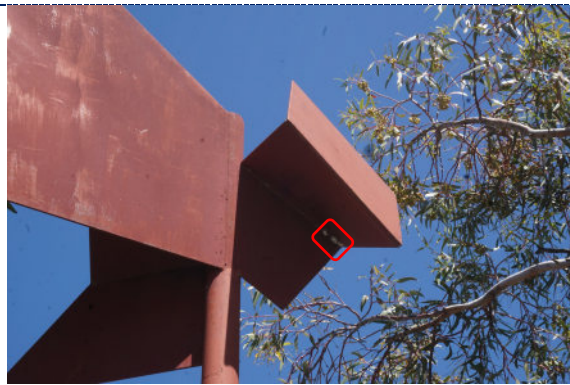
Figure 5: Detail – paint chalking, overpaint; spider webs.
