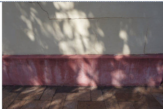
Figure 5: Detail – surface cracks and deformation to the mortar; chalking (UV degradation) and fading of the paint; staining to the exterior of the cracks.
