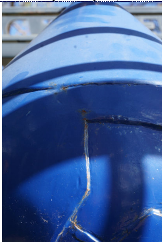
Figure 8: Detail – blanching of blue paint layer, appearing as white hazy bloom on upper section of 'drop' component. Minor losses and areas of corrosion also visible.
