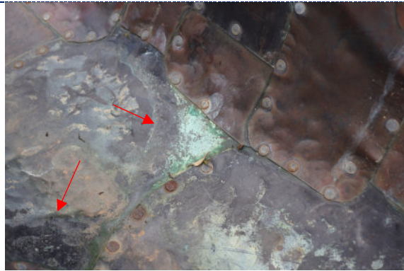
Figure 23: Detail – interior, dirt particulate, green copper corrosion in areas where water pools.
