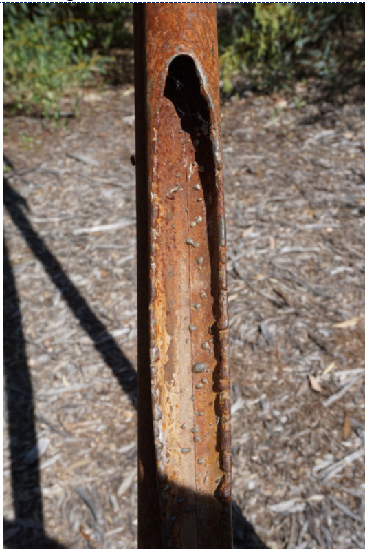
Figure 9: Detail – dirt particulate; surface corrosion.
