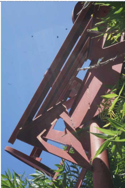
Figure 11: Detail – paint chalking, flaking, overpaint; surface corrosion; woody plant growth interaction.
