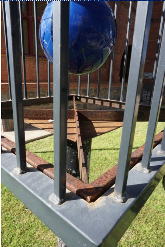
Figure 5: Detail – extensive corrosion of steel in cross-bar mid section base.
