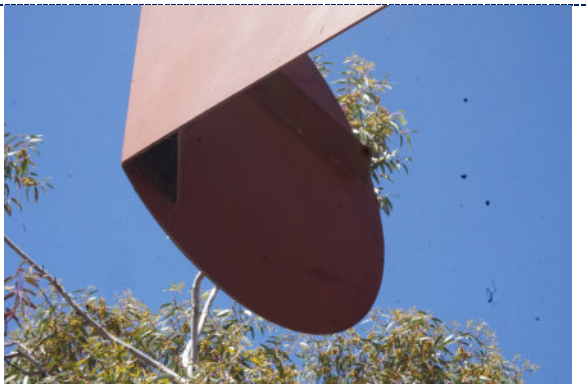
Figure 12: Detail – f paint chalking, overpaint.
