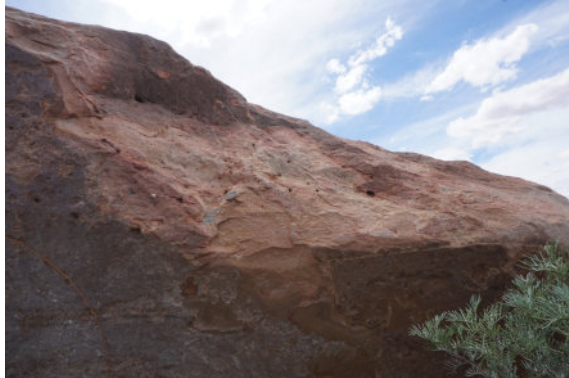
Figure 17: Detail – possible stone delamination.
