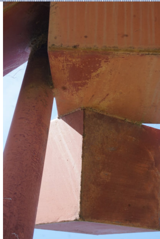
Figure 16: Detail – paint chalking, flaking paint loss; spotted surface corrosion.
