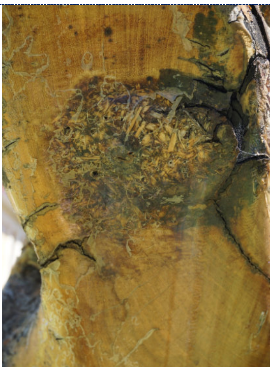
Figure 17: Detail – exterior-bottom, degraded and peeling varnish.
