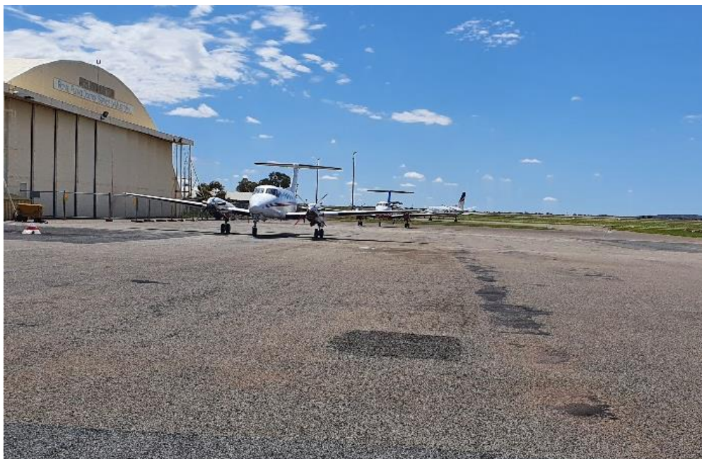
Figure 18: RFDS Apron showing patched pavement
