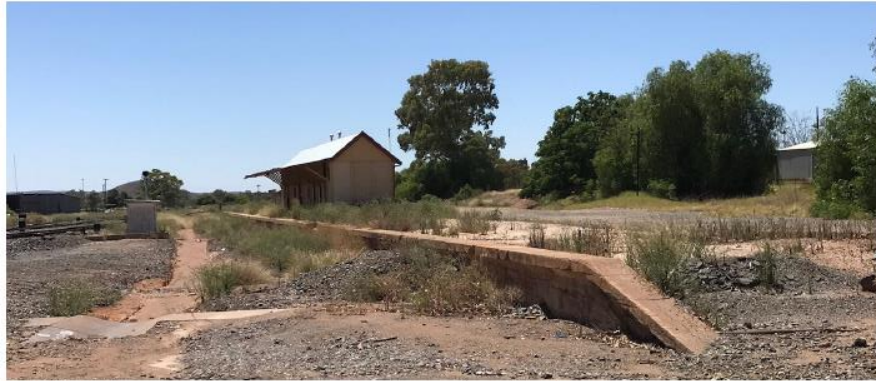
The Old Railway station surrounds - note poor condition of platform and road
